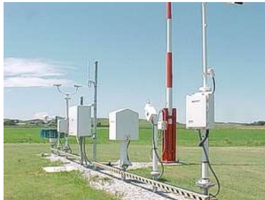
Figure 2-5: Typical Airport ASOS Station
