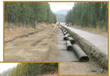
SSDL installed on the northbound lane
