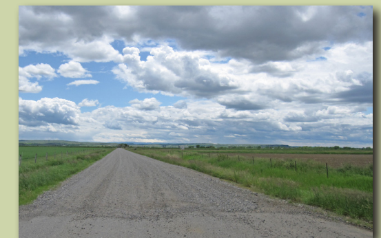
This segment of Five Mile Road would be improved under all build alternatives
