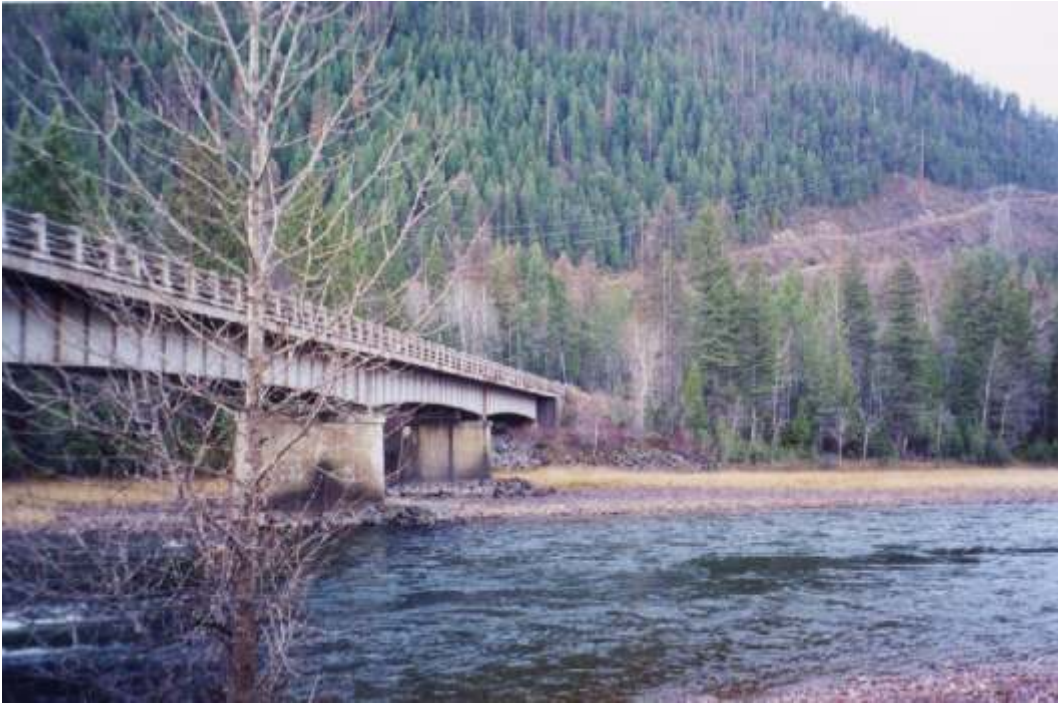
Existing South Fork Bridge west of Hungry Horse. Photo taken looking southwest from approximate location of proposed new bridge.
