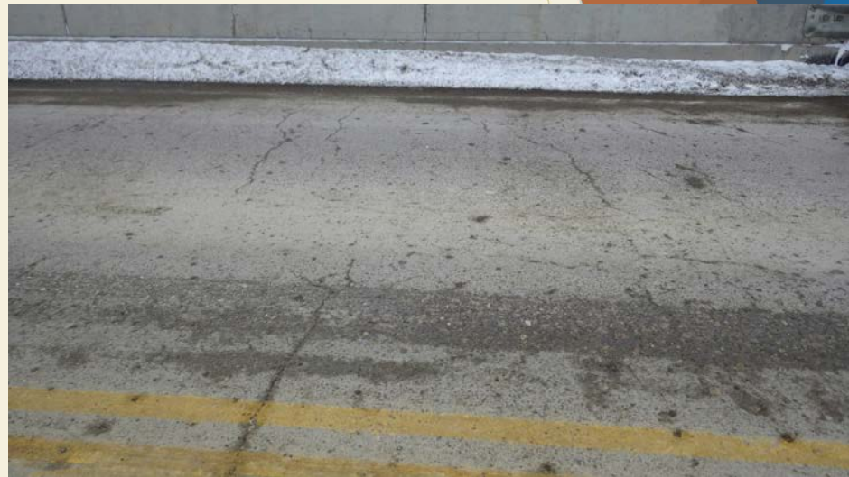
Image of Deterioration to Bridge Deck
