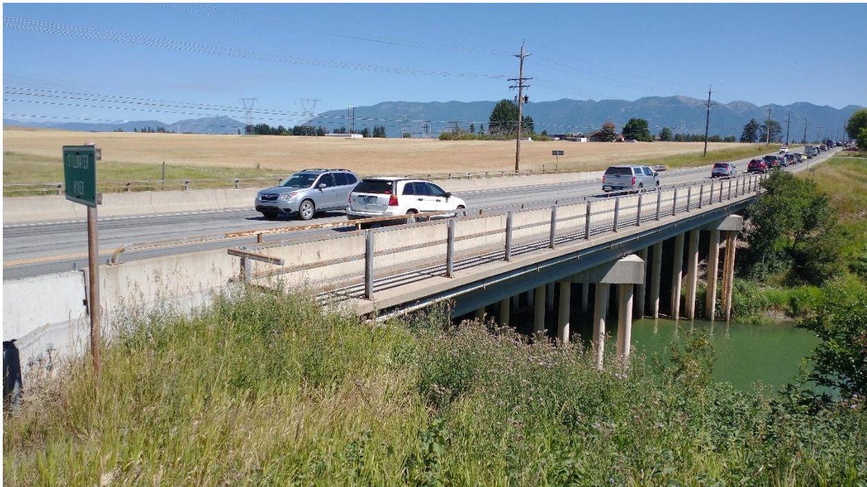
The two bridges in the study area are currently in need of repair, maintenance, or replacement.
