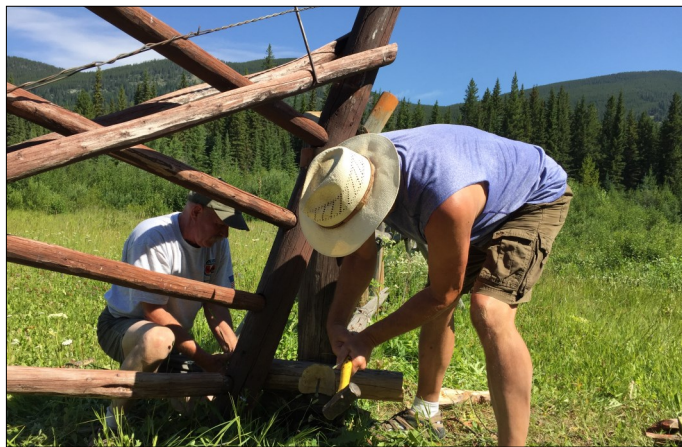
Lynn Kleen, of Stevensville, and Jim Brown, right, of Billings make repairs to the gate on the east end of the field.
