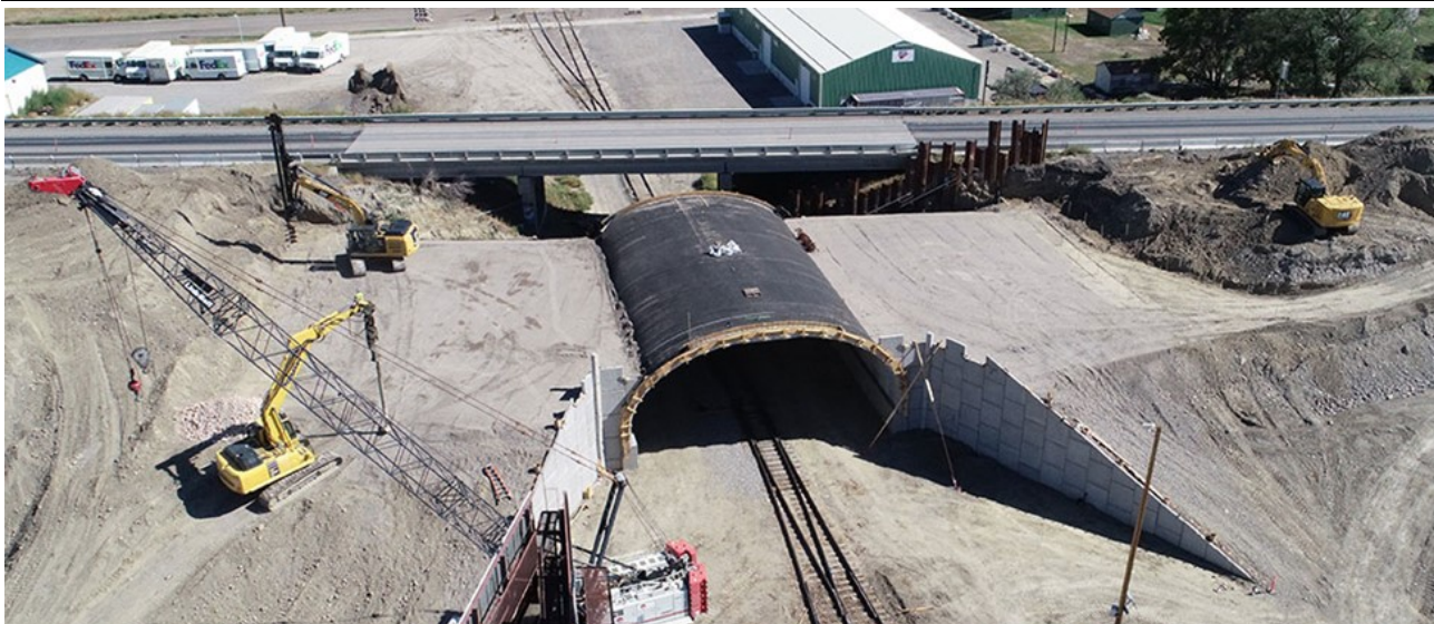
Drone footage of the I-90 Yellowstone River—Billings Project in 2022. This project includes reconstruction of the 1000-foot-long bridges over the Yellowstone River and the Talen Energy railroad spur line, and is tentatively scheduled to be completed in 2024.
