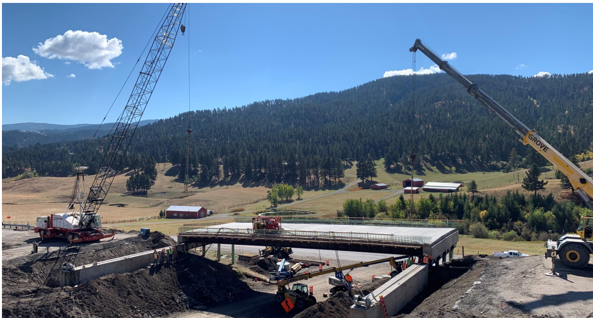
Progress on the I-90 Quinn Creek Road Bridges Project between Livingston and Bozeman in the summer of 2022. The photo shows the eastbound bridge deck cast off the alignment and the new foundations that the deck cast would eventually be rolled onto. This illustrates the Accelerated Bridge Construction (ABC) method used at this stage of the project. ABC methods allowed crews to advance multiple elements of the project simultaneously to ultimately expedite project completion.
