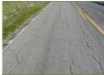
Prevalent cracking in extent and severity, heavy rutting, patching
