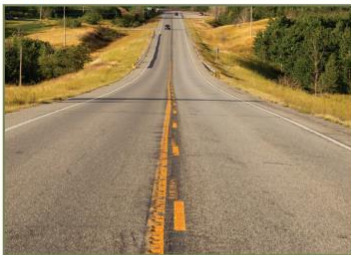
Moderate cracking in extent and severity, slight rutting and aggregate loss
