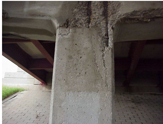
Figure 34: Deteriorated column of I-96 overpass bridge, Michigan [42].
