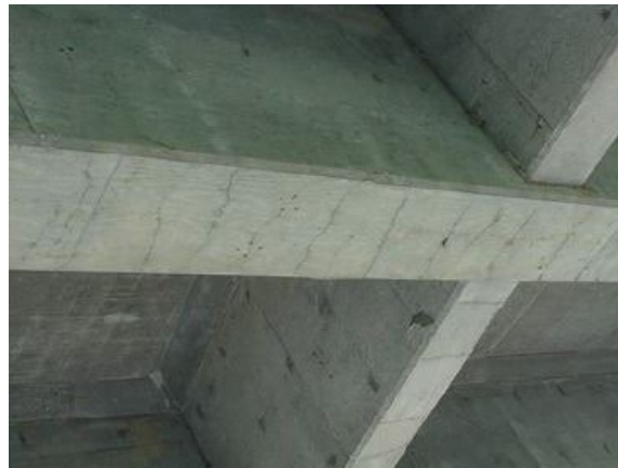
Figure 27: Cracks in Louisa Fort Gay bridge [39].
