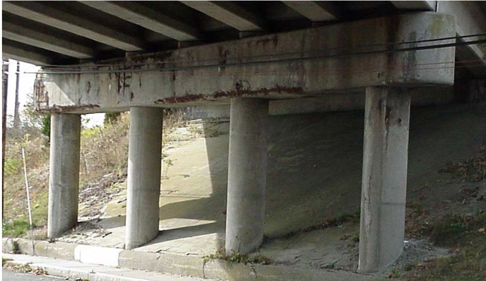
Figure 37: Deteriorated pier cap of Salt Pond Road Bridge [44].
