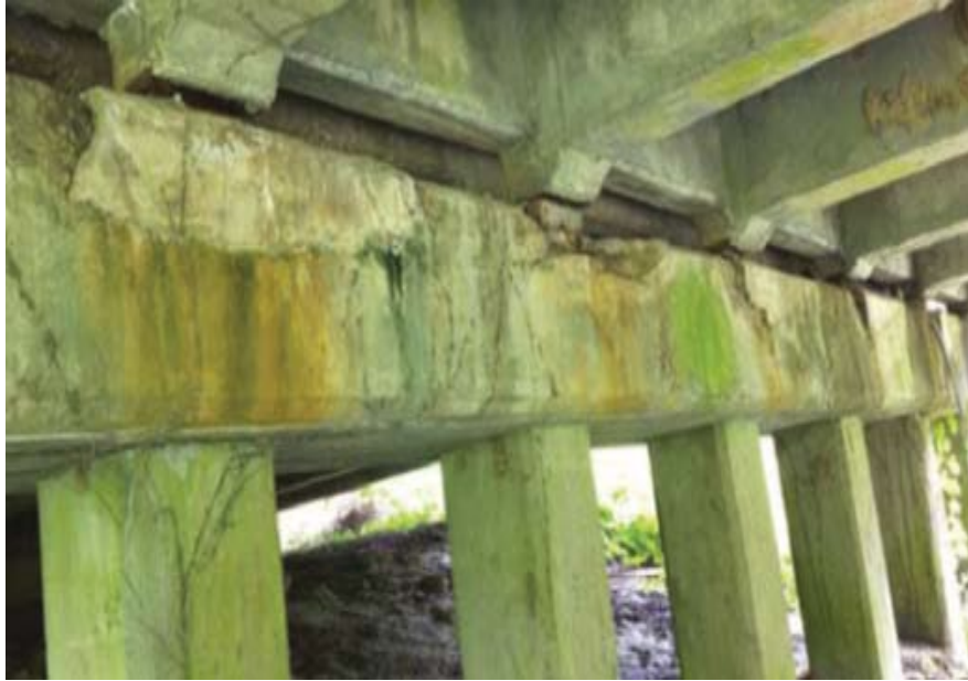
Figure 40: Delamination under the bearing plate of the Morganza Spillway bridge, Louisiana [45].
