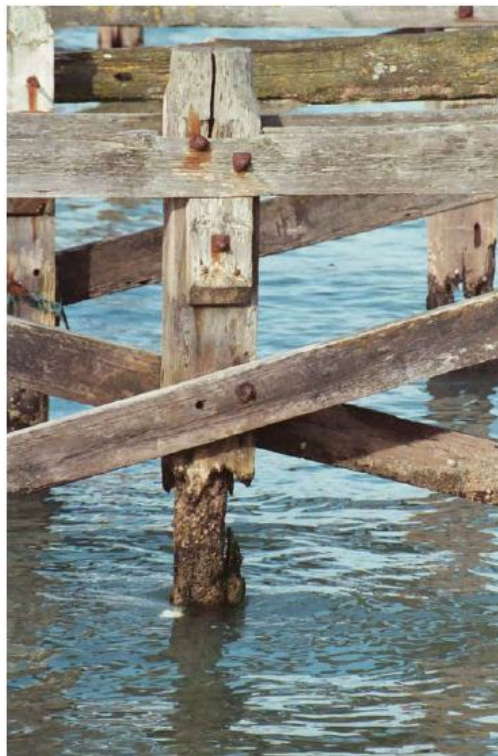
Figure 19: Biologically degraded pile [37].
