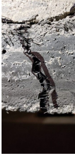
b) Crack progressing through UHPC with steel fibers spanning
