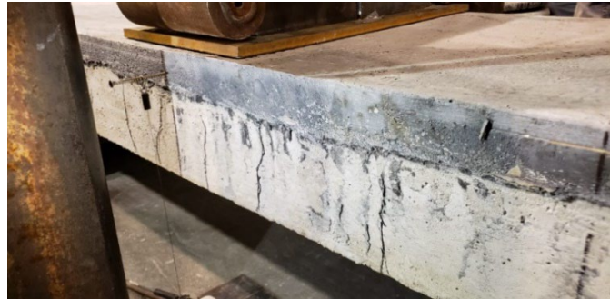
a) Flexural cracks initially forming
