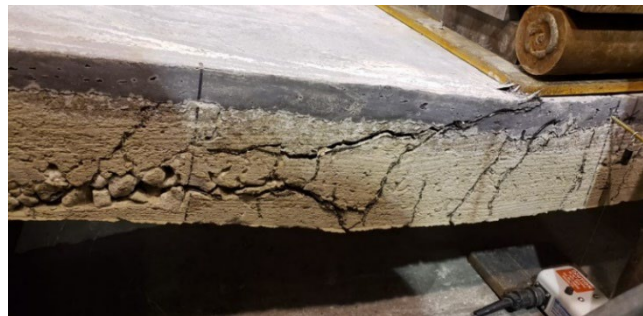
b) Shear crack on one end of slab
