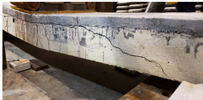
c) Shear crack formation
