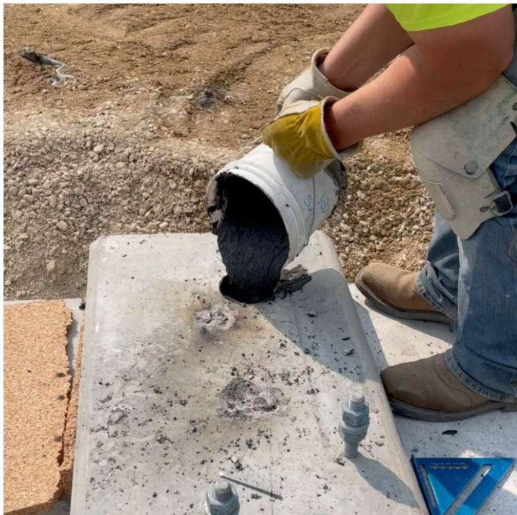
Figure 59: UHPC being placed into beam dowel hole, connecting it to pile cap
