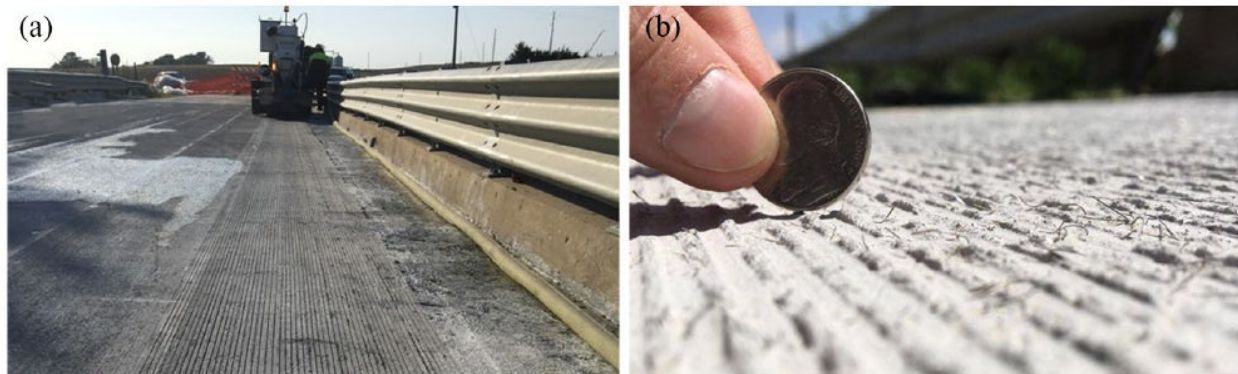
Figure 4: UHPC overlay on Mud Creek Bridge deck: (a) grooving of the surface; (b) closeup of finished surface [6]
