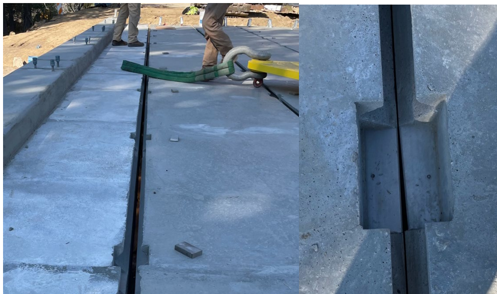
Figure 56: Shear tabs just prior to welding (left), and shear tab connection without tab (right)
