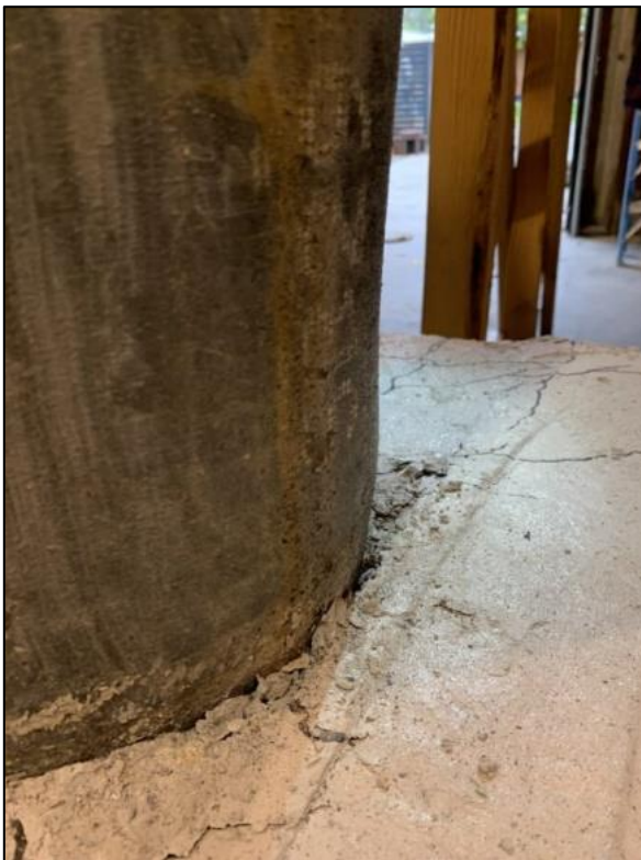
Figure 49: VT2/3-4U buckling of CFST after formation of plastic hinge initial pull direction
