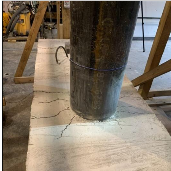
Figure 48: VT2/3-4U 45-degree cracks (184 k-ft)
