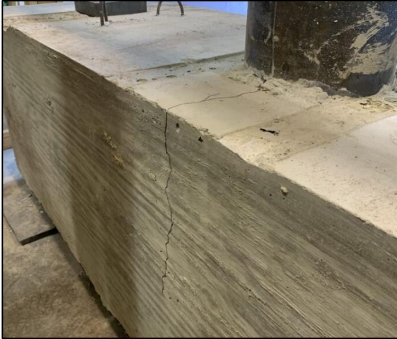
Figure 41: VT2/3-6 first cracks (69 k-ft)
