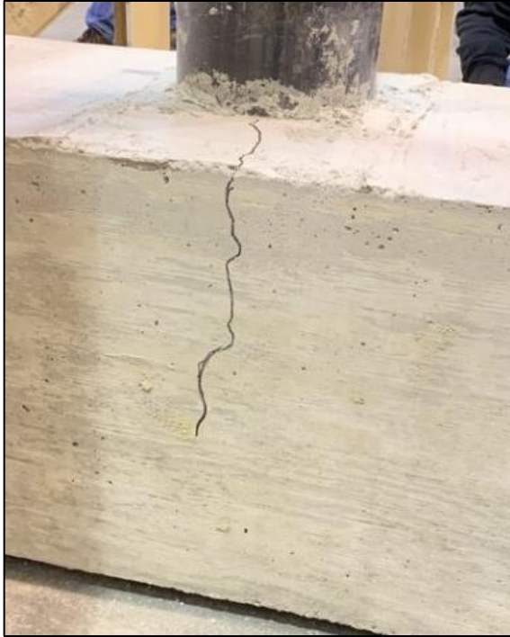
Figure 26: VT1/2-4 first cracks (47.3 k-ft)
