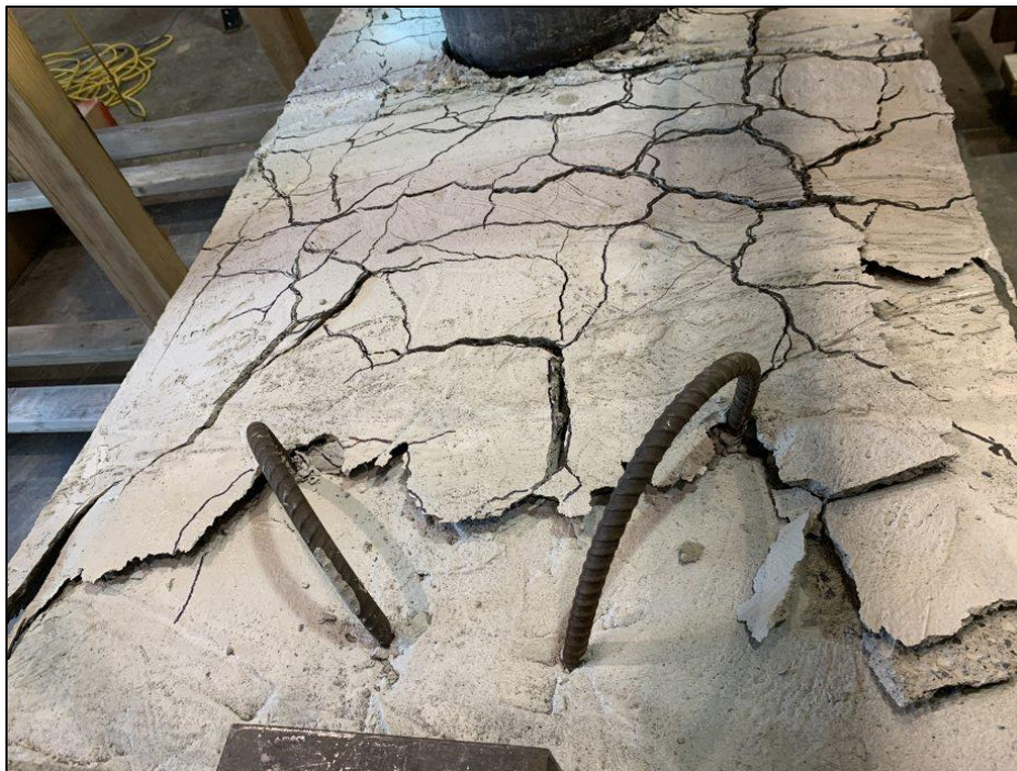
Figure 53: VT2/3-4U prying action on back side of pile cap
