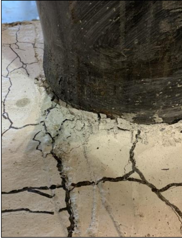
Figure 51: VT2/3-4U buckling of CFST after formation of plastic hinge reverse push direction
