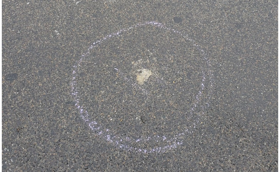
Delaminated area identified on Bridge 3734
