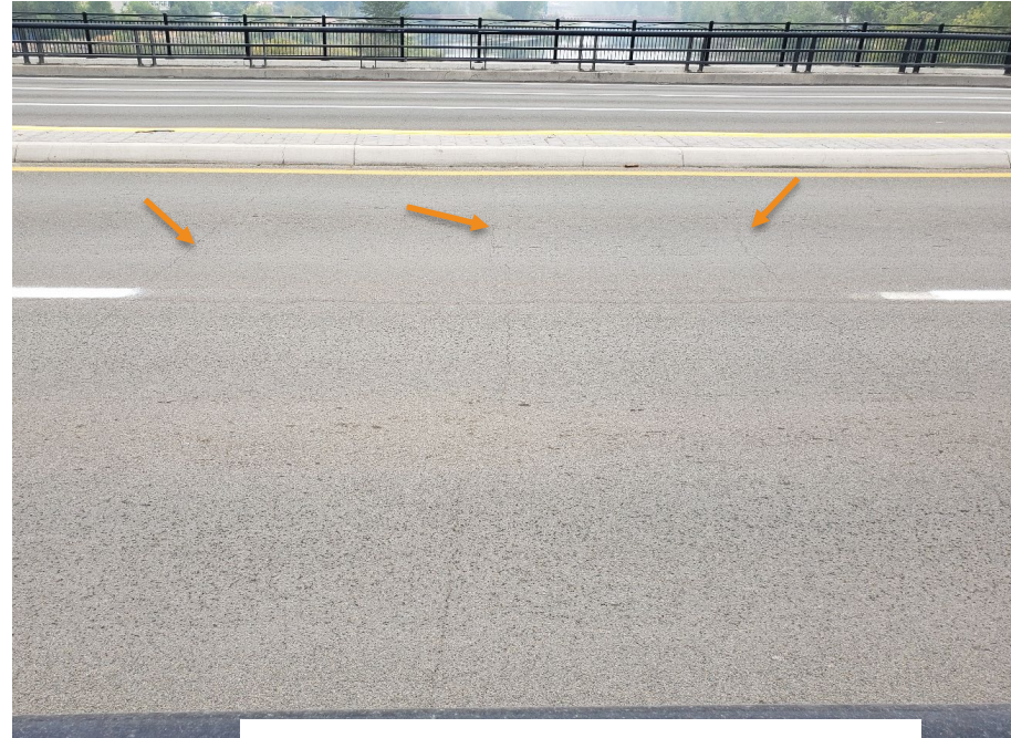
Transverse cracking in 14/25
