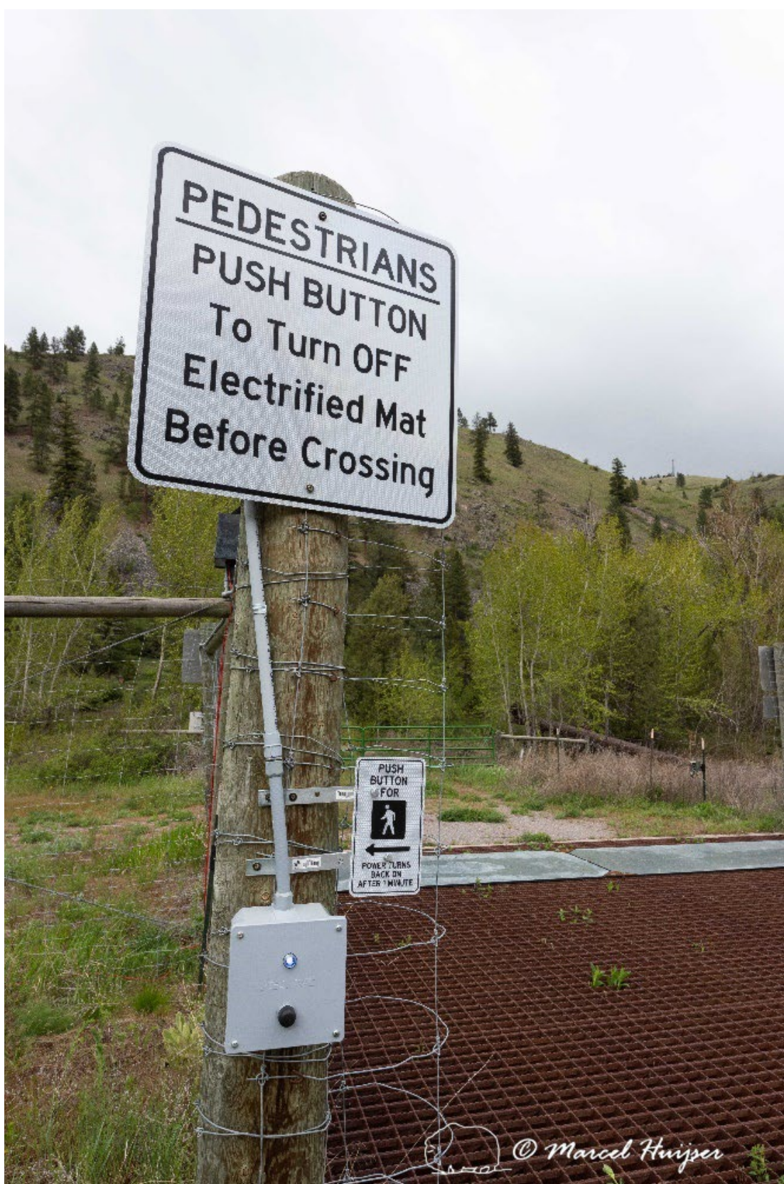
Figure 6: Push button for pedestrians to temporarily (about 1 minute) turn off the power.
