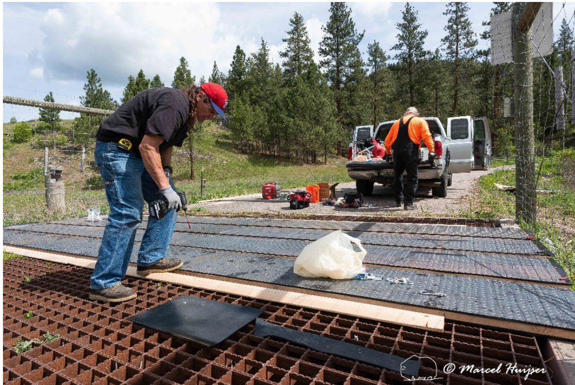
Figure 2: The installation of the electrified mat by Crosstek at the north wildlife guard, US Hwy 93, south of Ravalli, Montana.
