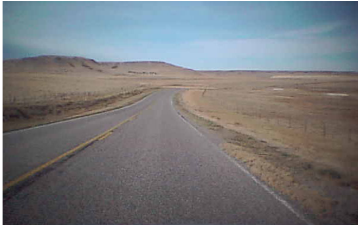
Photo 1-4: View of narrow roadway and lack of shoulders.
