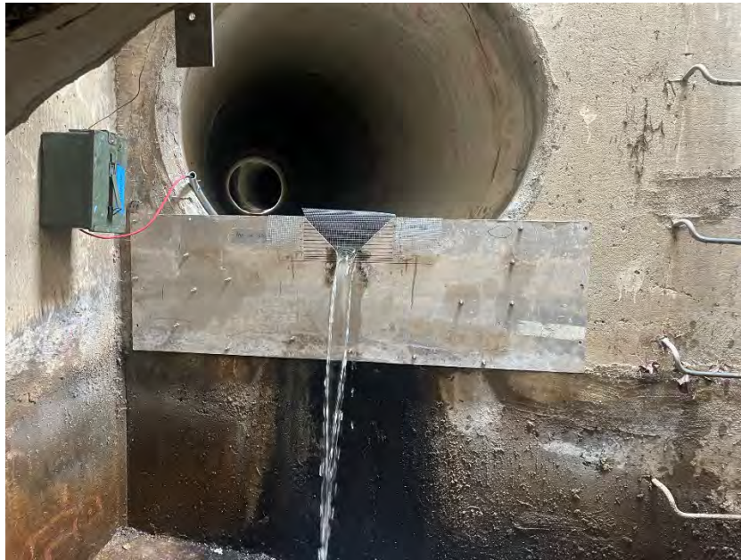
Figure 4-2. V-notch Weir on Outfall
