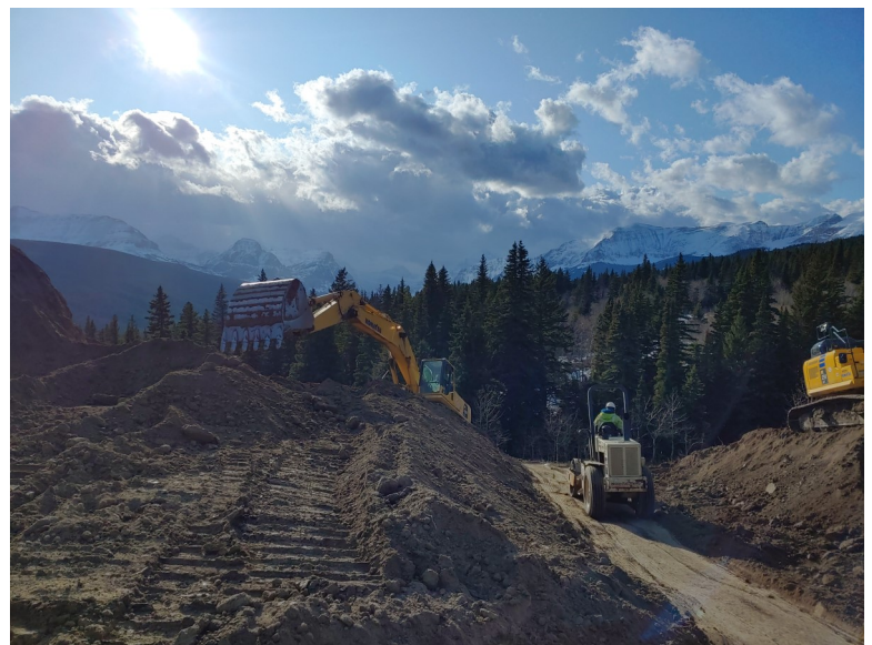
Active construction on the North of Kiowa North project near Browning, Mont. (featured on Page 1)
