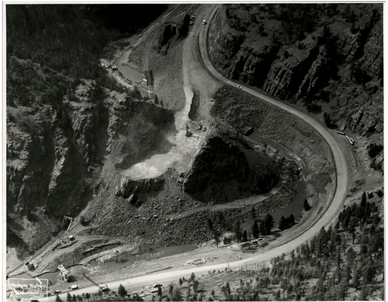
An aerial photo shows highway construction at the south entrance of the canyon.
