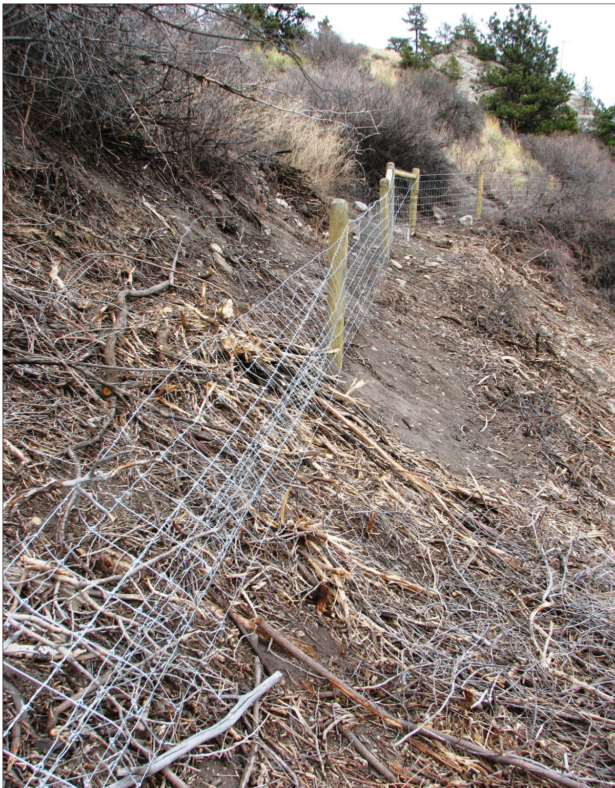
↑ View north of damaged fence section.
