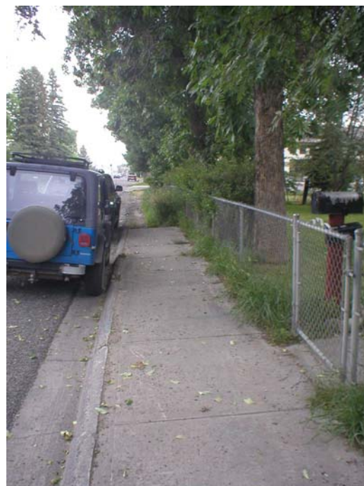
Photo 1-1 Discontinuous sidewalk along Rouse
