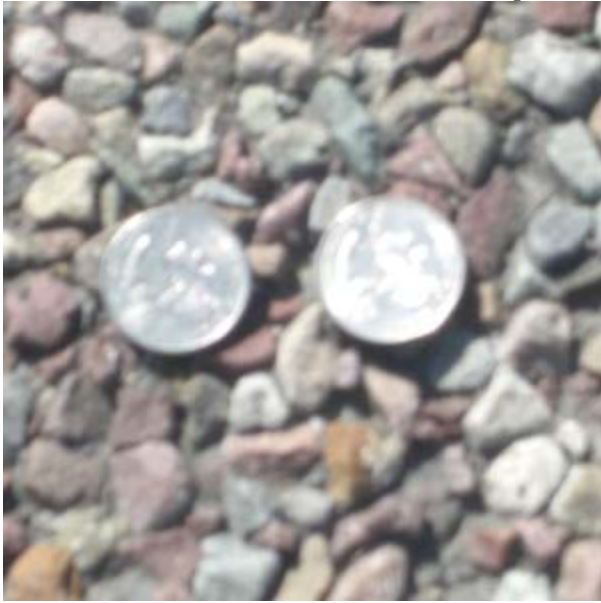
(c) Site 14 (P-52), Failed Chip Seal
