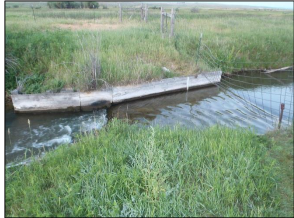
Photo 2. Parshall flume used to measure Co-op Ditch flow
