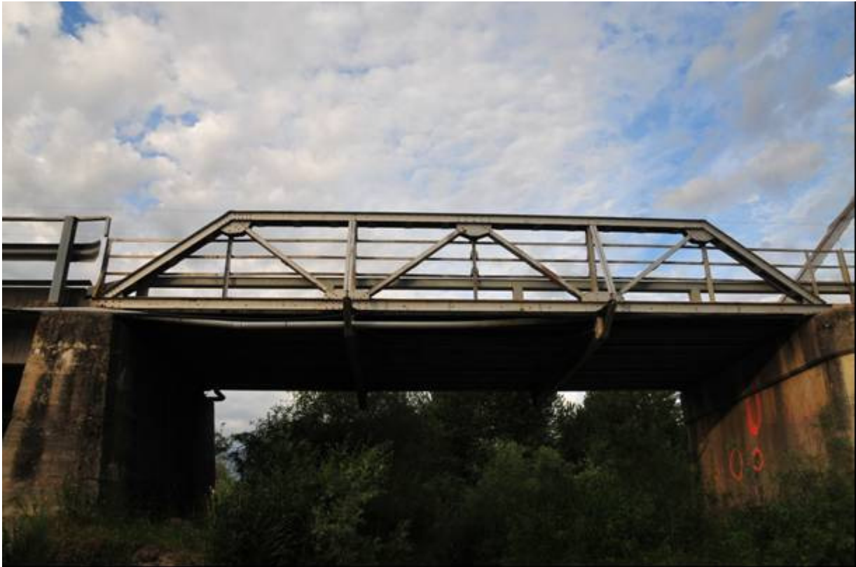
Photo MT_MissoulaCounty_MaclayBridge_0005 (5 of 9) - Maclay Bridge: view to the southwest showing the Warren pony truss with the circa 1923 solid reinforced concrete pier to the right and possibly circa 1953 pier to the left.
