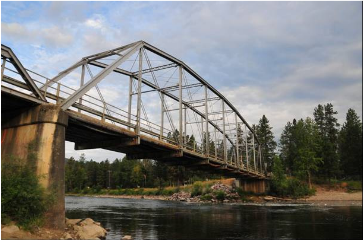
Photo MT_MissoulaCounty_MaclayBridge_0006 (6 of 9) - Maclay Bridge: view to the west showing the riveted Parker through truss component. Concrete abutment with wing walls on the west bank of the river / solid reinforced concrete pier at the junction of the through-truss and pony-truss components.
