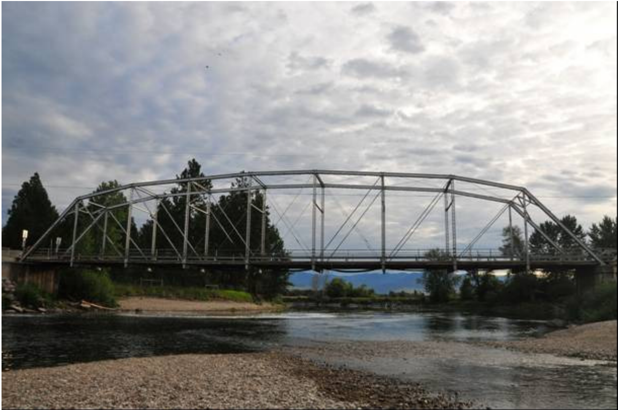
Photo MT_MissoulaCounty_MaclayBridge_0009 (9 of 9) - Maclay Bridge: view to the north showing the panels, channels sections, and angle sections of the riveted Parker through truss span.
