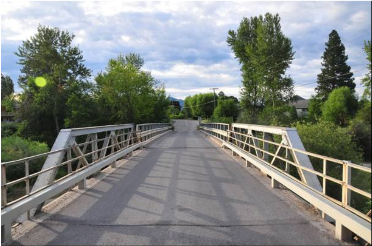
Photo MT_MissoulaCounty_MaclayBridge_0007 (7 of 9) - Maclay Bridge: view to the southeast across the deck of the Warren pony truss component and of the pre-stressed concrete approach spans with high steel I-beam guardrails.
