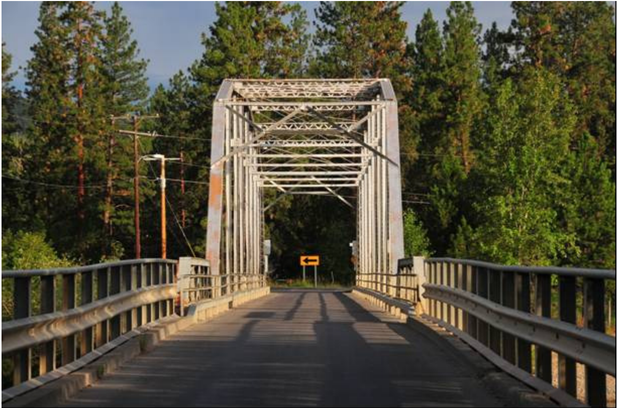
Photo MT_MissoulaCounty_MaclayBridge_0008 (8 of 9) - Maclay Bridge: view to the northwest across the bridge deck.
