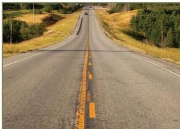
Moderate cracking in extent and severity, slight rutting and aggregate loss
