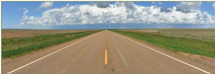
Visible traffic wear with low severity cracking and minimal rutting
