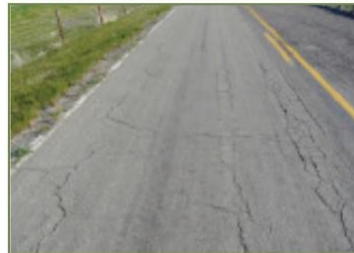
Prevalent cracking in extent and severity, heavy rutting, patching
