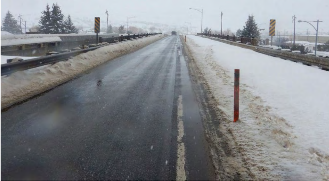
Figure 4.1-1 A follow-up inspection is required to check the condition of the bridge deck and associated elements (joints, rail, etc.).
