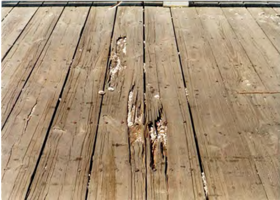
Figure 5.6-1 Deterioration of timber plank deck surface.
