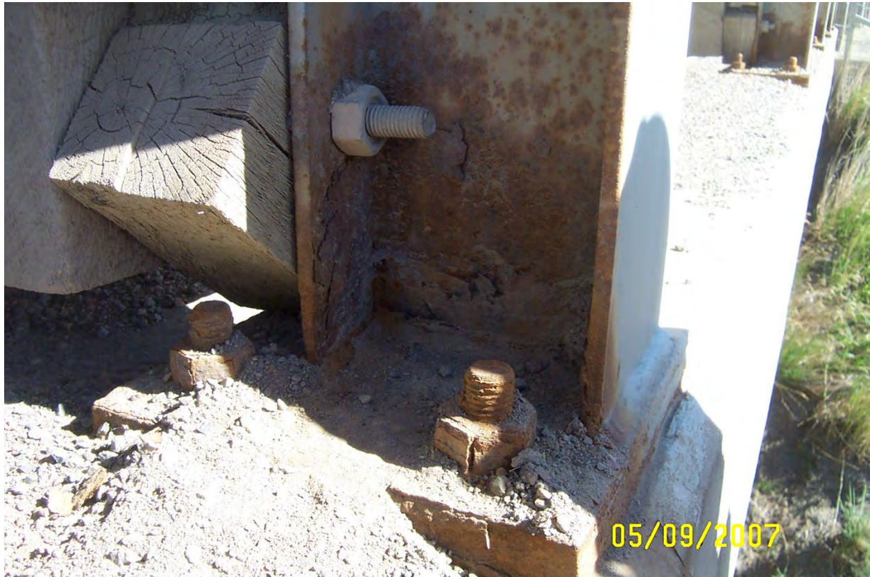
Figure 5.6-9 Steel Bridge Railing Post with Corrosion
