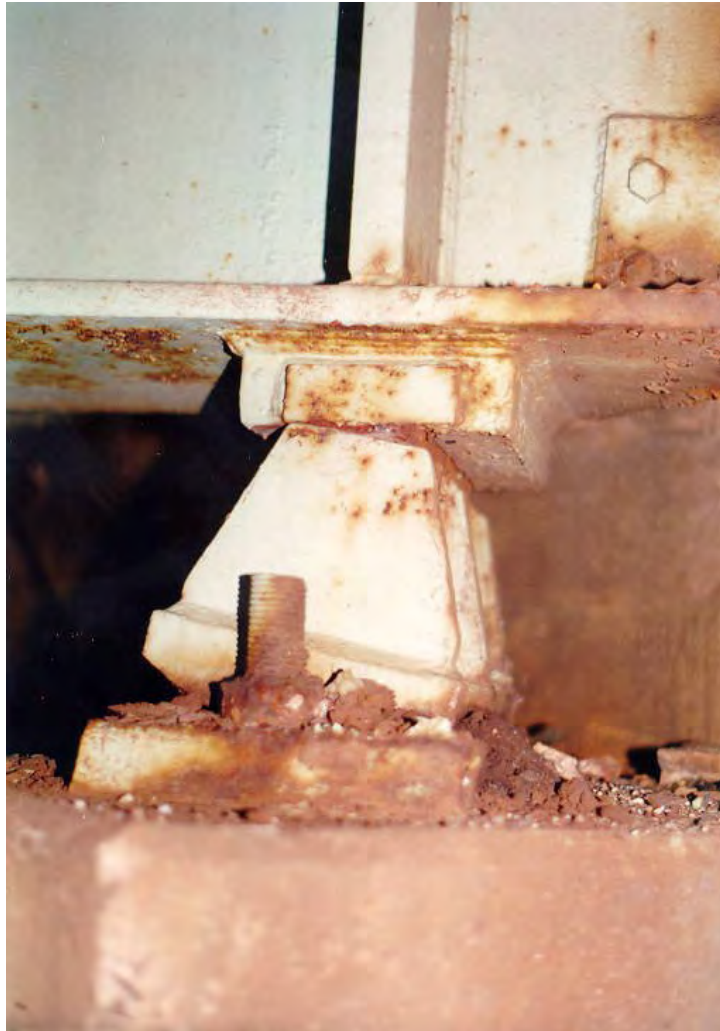
Figure 5.7-9 Over Extended Rocker Bearing.
