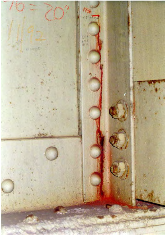
Figure 5.7-29 Fatigue Crack in a Diaphragm Connection Angle on a Girder.
