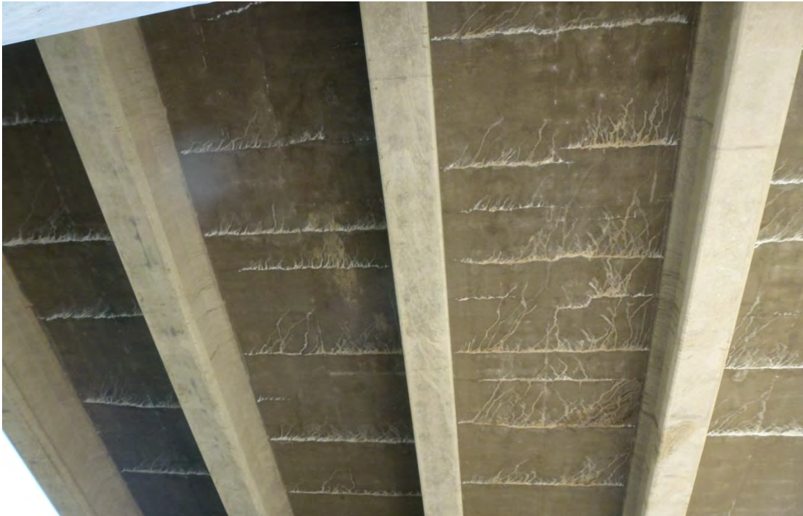
Figure 9. Example of Condition State 3. Note the tight spacing (12" to 18") of some of the transverse cracks, along with evidence of heavy leakage and some gray efflorescence. Also, small jump cracks are evident.
