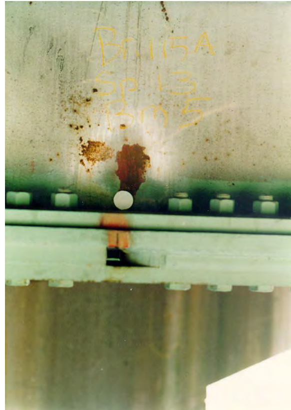
Figure 5.7-28 Fatigue Crack Through the Bottom Flange of a Rolled Stringer at the End of a Partial Length Welded Cover Plate. (A stop hole has been drilled in the web and splice plates have been bolted to the bottom flange.)
