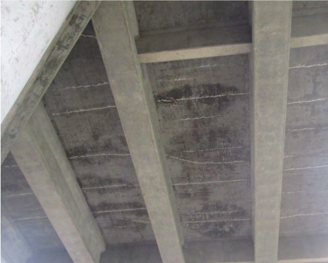
Figure 3. Typical Transverse Cracks Seen from Underneath.
