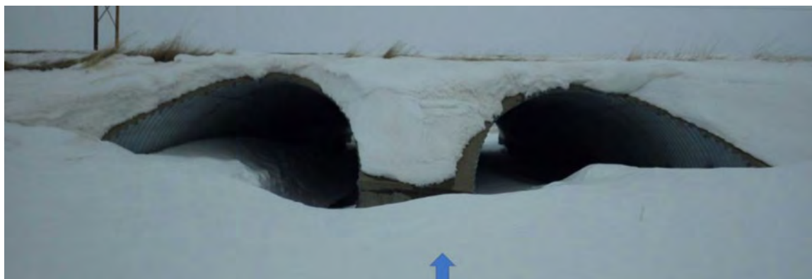
Figure 4.1-4 A follow-up inspection is required to check the condition of the pipe culverts.
