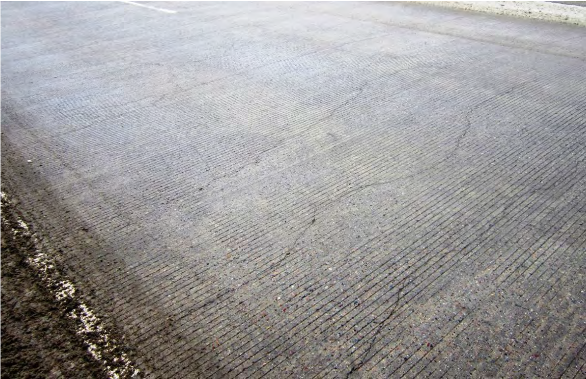
Figure 2. Transverse Cracks in Bridge Deck
