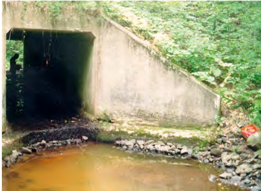
Figure 5.10-1 Cast-In-Place Concrete Culvert with Erosion at the Outlet.
