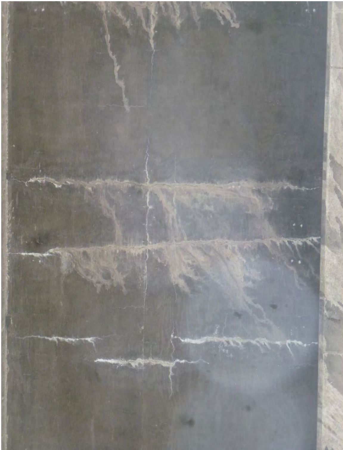
Figure 6. Example of Heavy staining from water leakage. (Note the contrast between the gray efflorescence in the upper 2 transverse cracks (evidence of concrete movement around crack and heavy water leakage and the white efflorescence in the bottom transverse cracks. Also note the longitudinal jump crack with light white efflorescence.)
