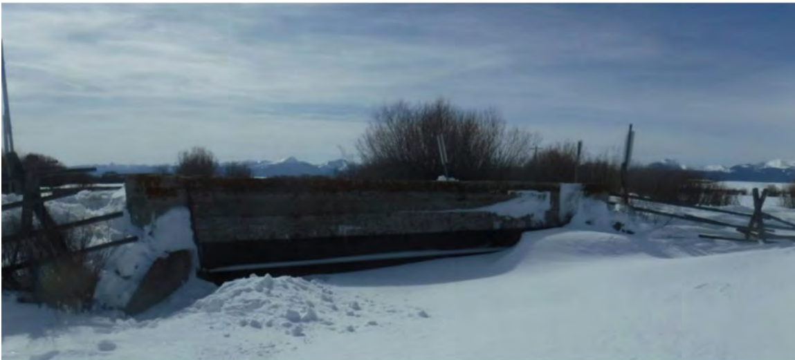
Figure 4.1-2 A follow-up inspection is required to check the condition of the wingwalls, abutments, and part of the exterior girder.
