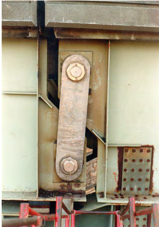
Figure 5.7-18 New Stainless-Steel Pin and Hanger with “Catchers Mitt” Retrofit Support Beam Installed.
