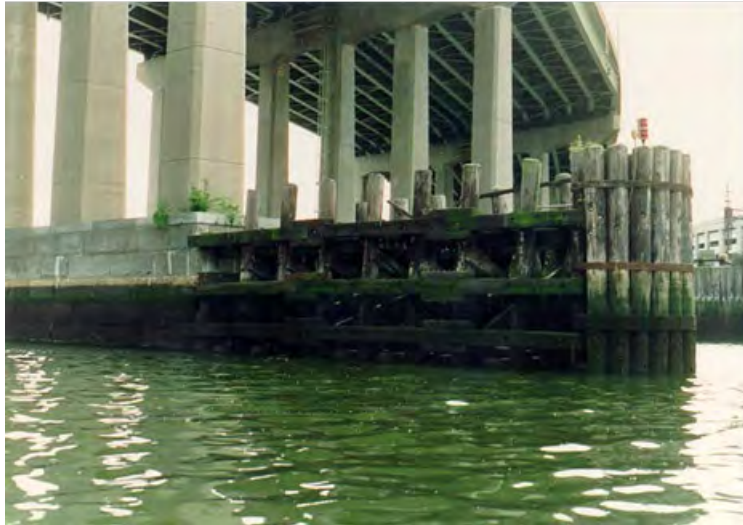
Figure 5.9-1 Timber Fender System with Navigation Lights.
