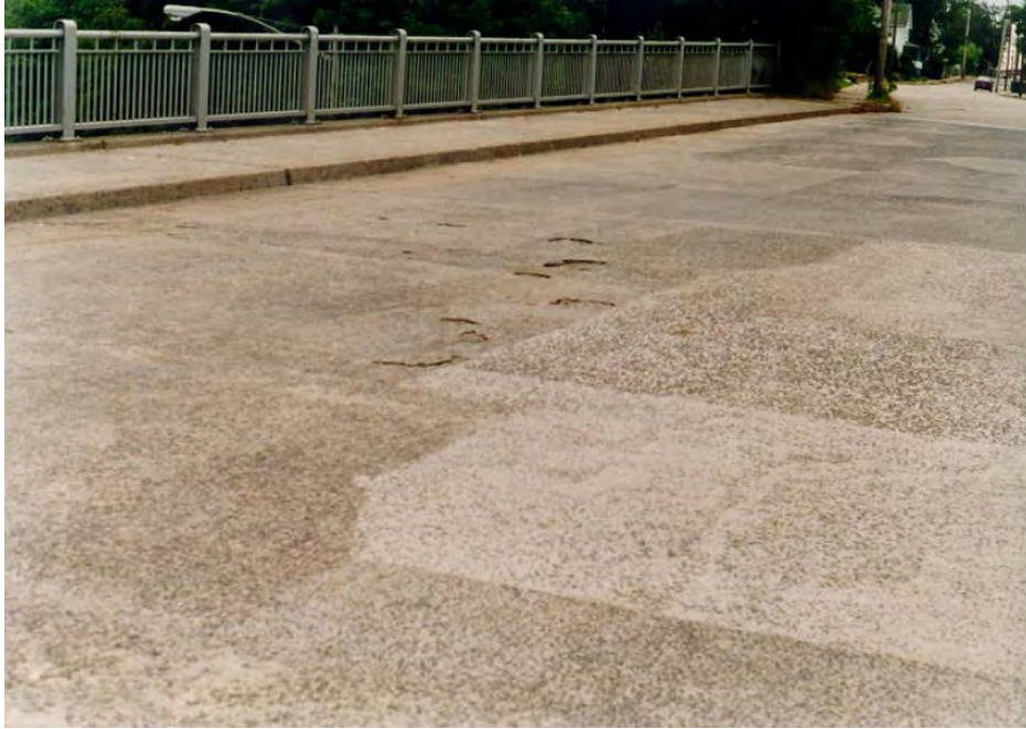
Figure 5.6-2 Top of Bare Concrete Deck with Patched, Spalled and Hollow Areas.
