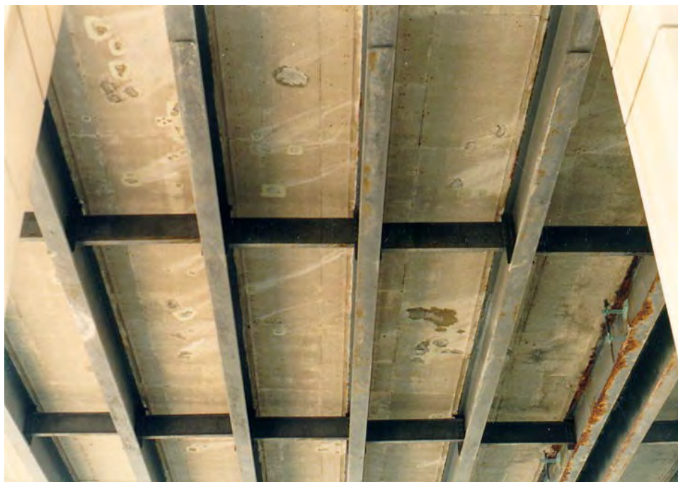
Figure 5.7-27 Typical Rolled Multi-Stringer Superstructure with Ends of Partial Length Welded Cover Plates Visible.
