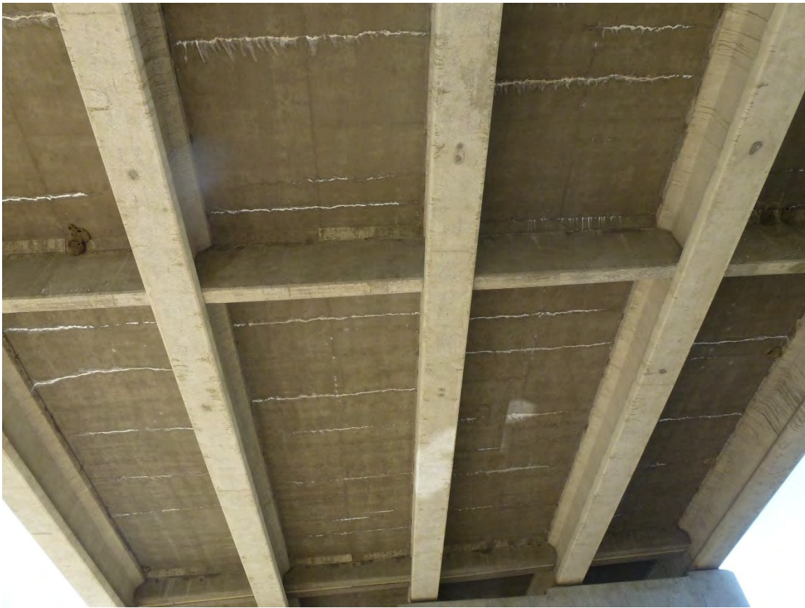
Figure 7. When to not use jump cracking defect. Use the deck cracking defect only. Transverse cracking is present but sporadic. Note the wide crack spacing, the lack of staining, and no longitudinal jump cracks. All efflorescence is white.
