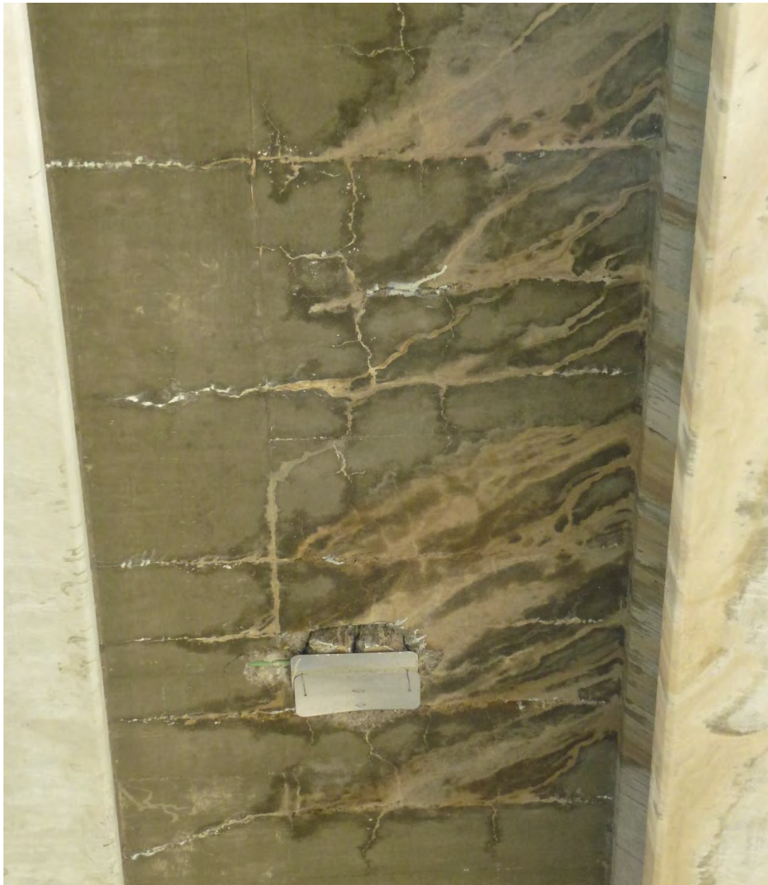
Figure 12. Example of Condition State 4. Tight spacing, jump cracks, “islands,” grey colored efflorescence present, very heavy water staining, repaired hole.
