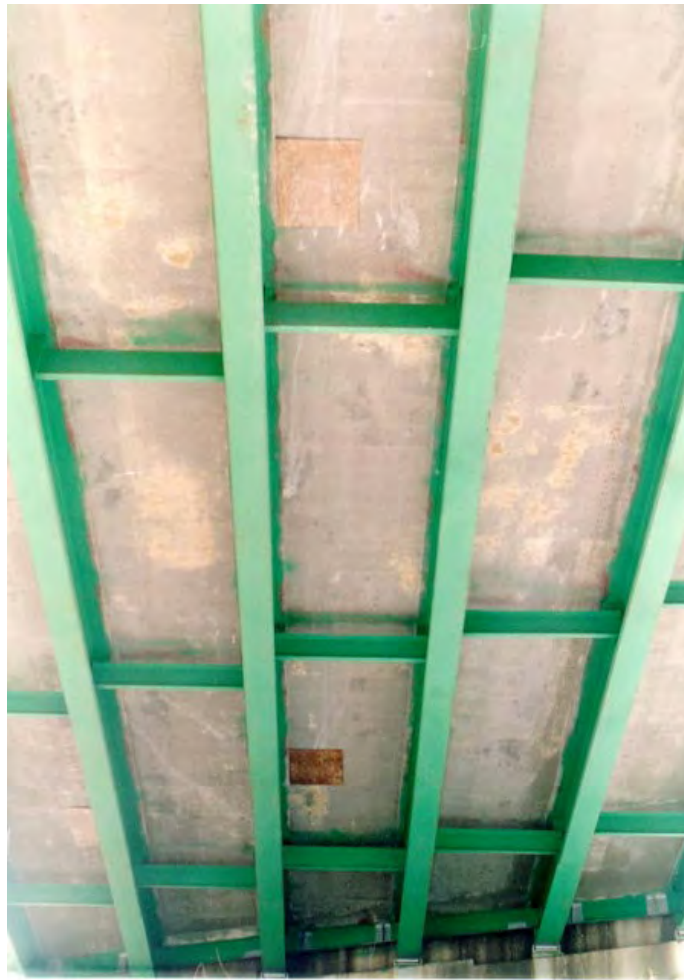
Figure 5.6-3 Typical Underside of Concrete Deck. Note Cracking with Efflorescence and Formwork Remaining from Full Depth Patching.
