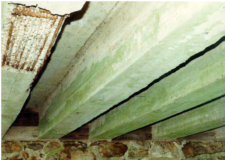
Figure 5.7-22 Concrete T-Beams with Large Spalls Exposing the Bottom Layer of Reinforcing Steel
