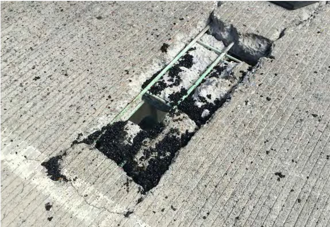
Figure 4 Holes in Bridge Deck. Note the longitudinal jump cracks that create the rectangular “island” of concrete. The “island” continued to crack until full depth chunk or “island” fell out, creating the hole.
