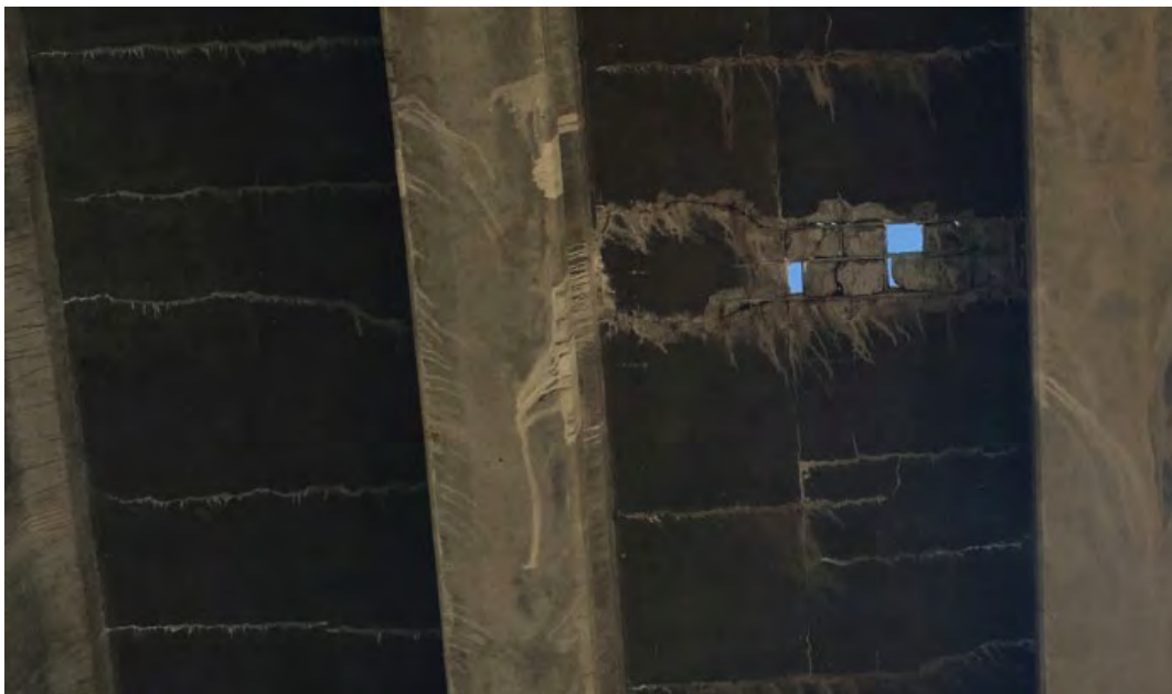
Figure 5. Same hole as Fig. 4 as seen from underneath. (Note the heavy staining on the soffit and girders from leakage in the cracks around the hole and in nearby transverse cracks and the jump cracks with staining beginning at another location not far from the hole. Also note that there are no jump cracks in the adjacent bay.)
