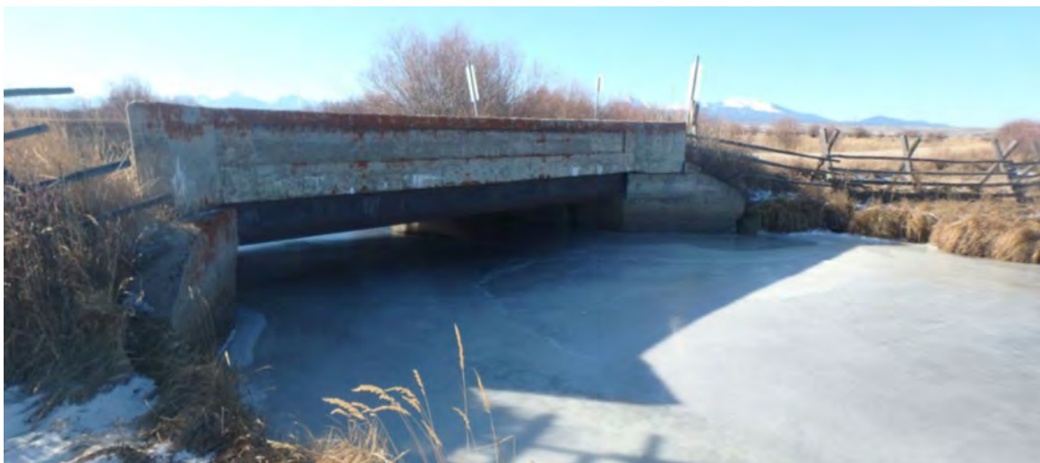
Figure 4.1-3 A follow-up inspection is required to check the condition of the bottom of the abutments and to check for scour.
