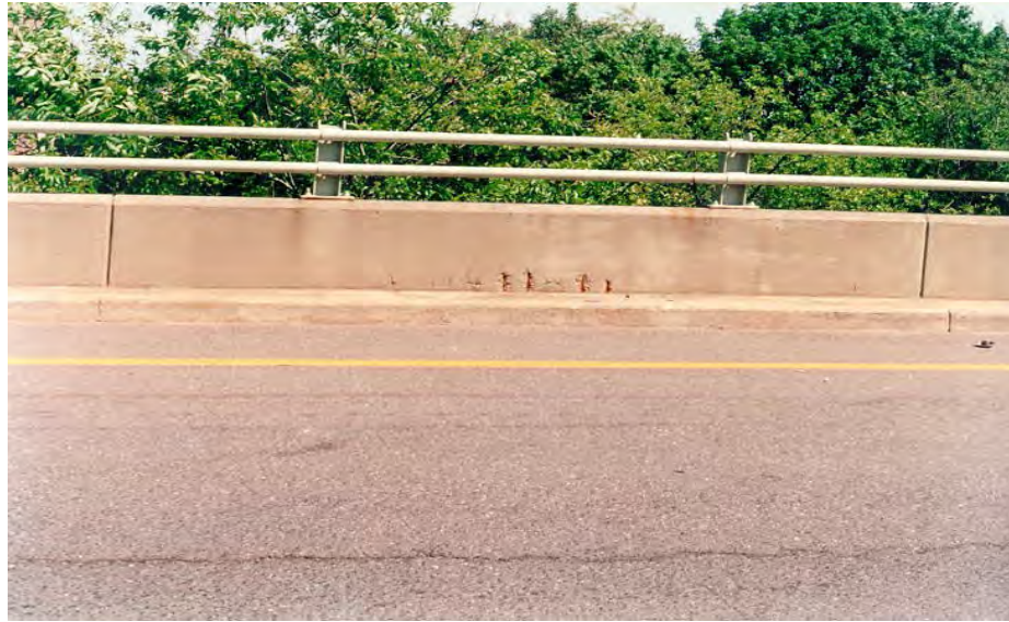
Figure 5.6-8 Concrete Parapet with Metal Pipe Railing. Note Spalling with Exposed Reinforcing Steel.
