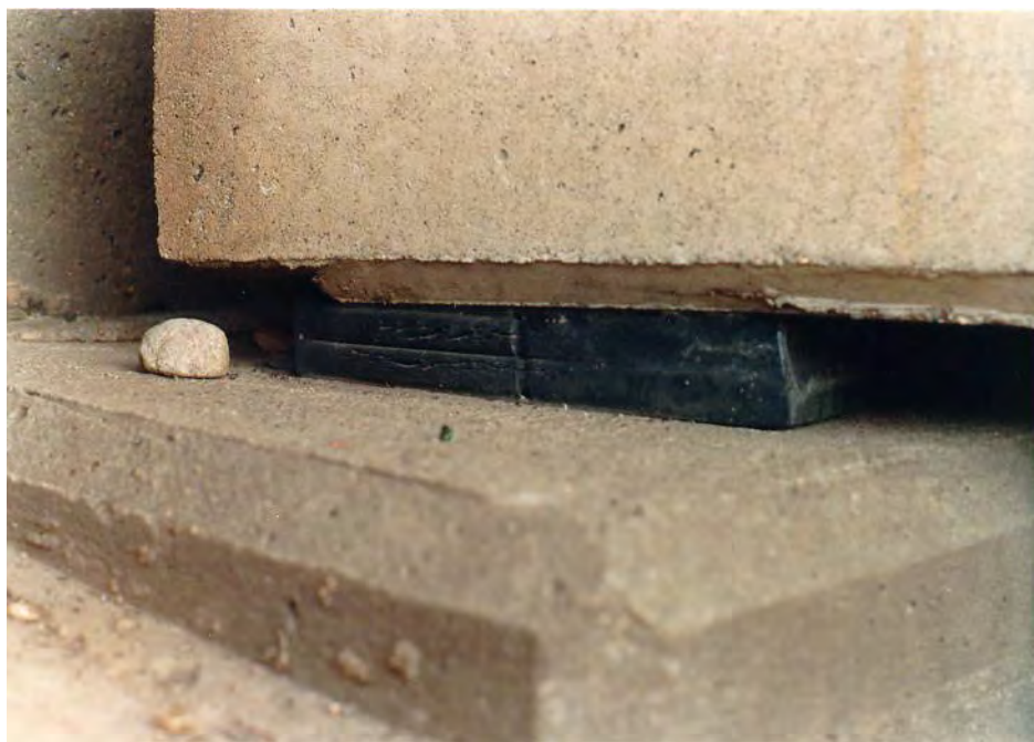
Figure 5.7-13 Elastomeric Bearing. Note the Non-parallel Bearing Surfaces
