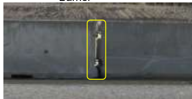
Missing connection pin NO TENSION
