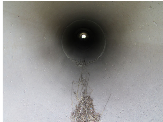
Figure 2: Inlet of pipe.
