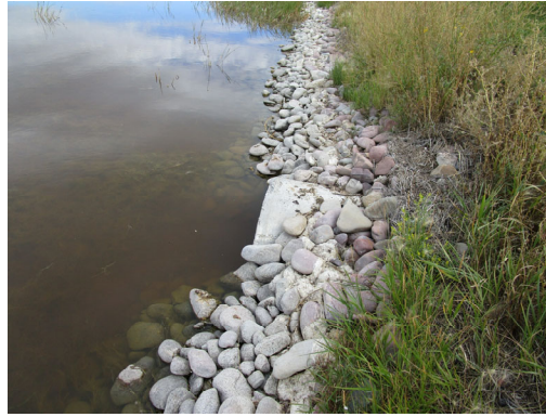
Figure 4: 36" RCP @ Basin Lake
