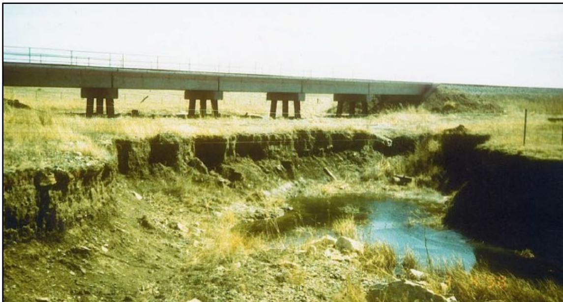
Figure 17.6-1 — HEADCUT DOWNSTREAM OF A BRIDGE
