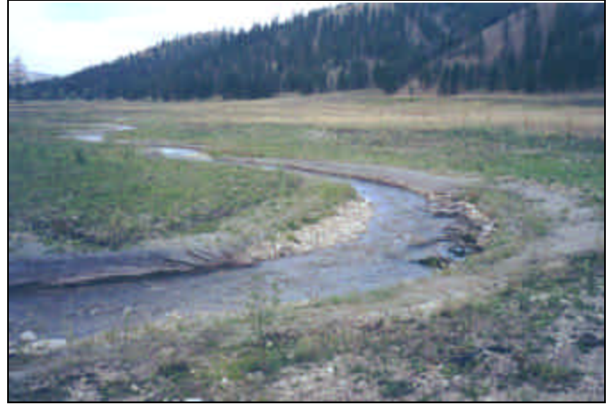
Photo Point No. 9: View looking north, main channel just below second culvert. Example of fabric work along constructed streambanks.
