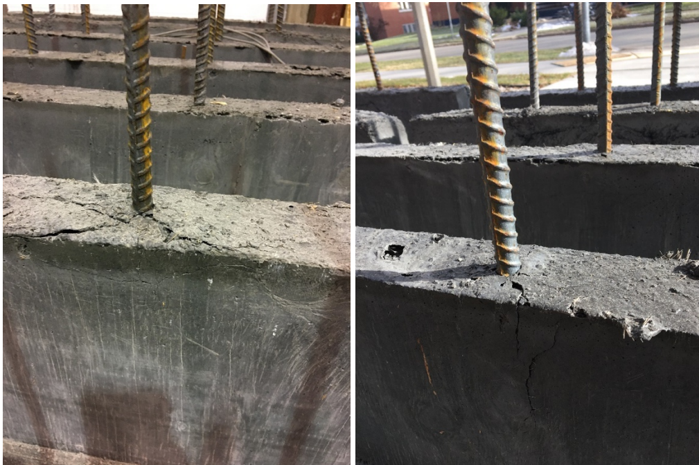
Figure 31: Bar Spacing test 7 showing UHPC splitting failure
