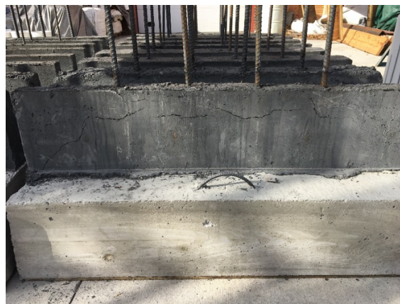
Figure 29: Side Cover tests 1 through 4 showing UHPC tension failure
