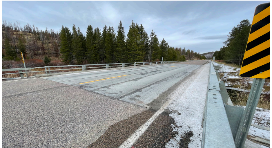
MDT used UHPC between the joints of precast concrete elements on this bridge replacement project.
