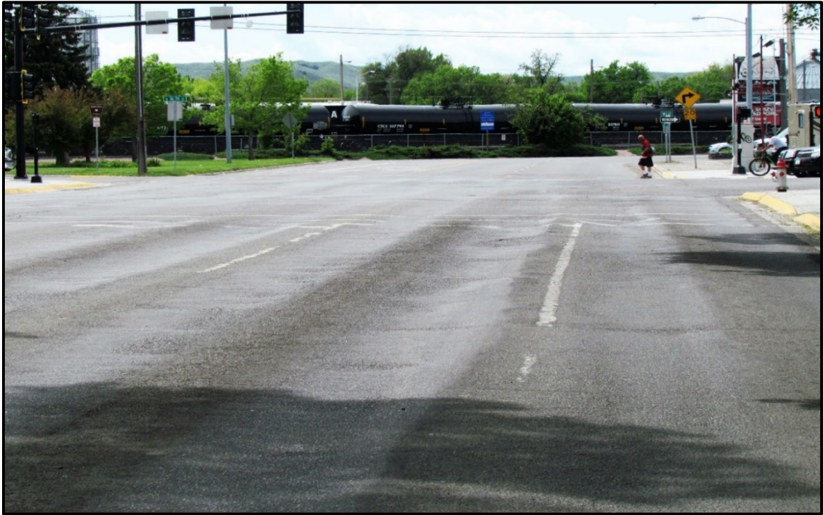
↑ Heavy rutting at the intersection of Division St. & Broadwater Ave. (view south).
