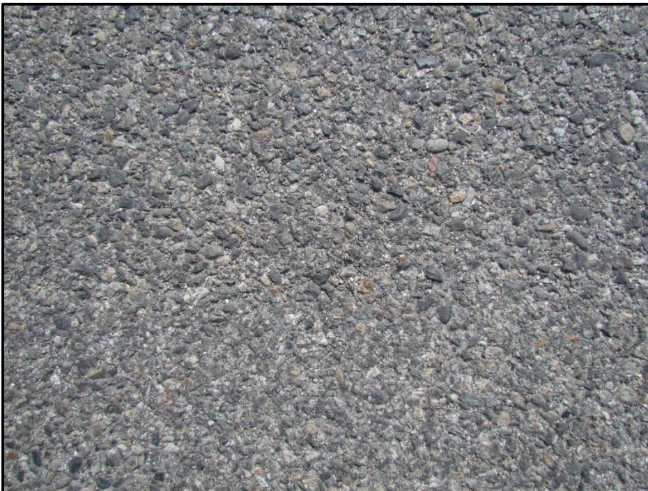
↑ Close-up of surface on Division St.
