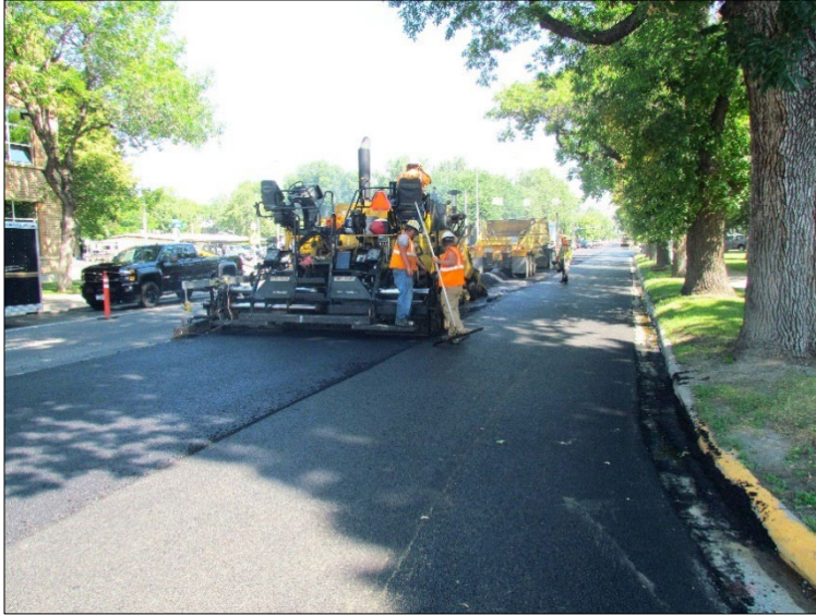
← Division St, view north. Representative image of the paving phase. The paver operators stated no perceived issues with the altered PMS during the paving process. Workers handling rakes at the paving edges did state the mix felt somewhat sticky.
