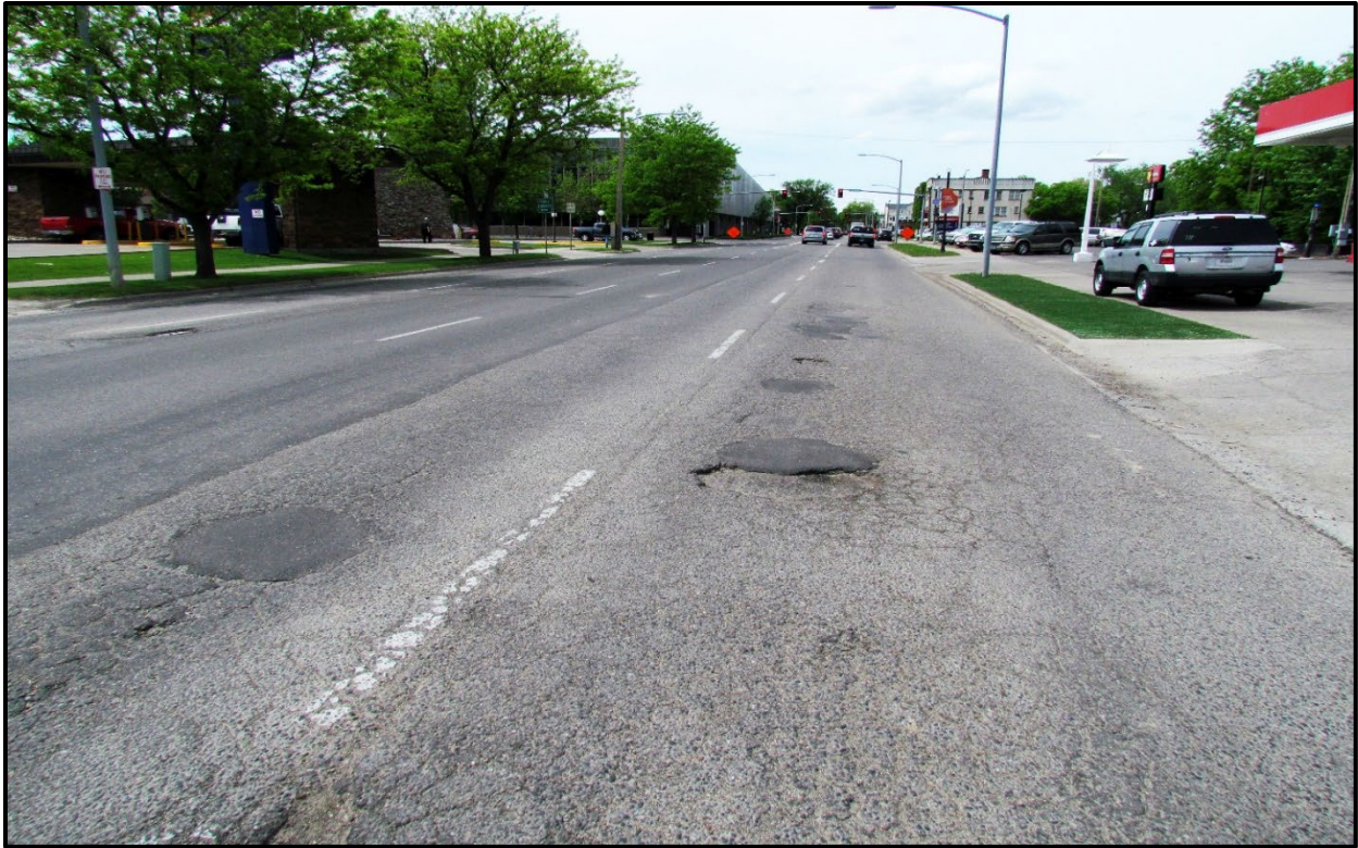
↑ Pavement distress on 6 th Ave N. specifically fatigue cracking and previous patching (view west).
