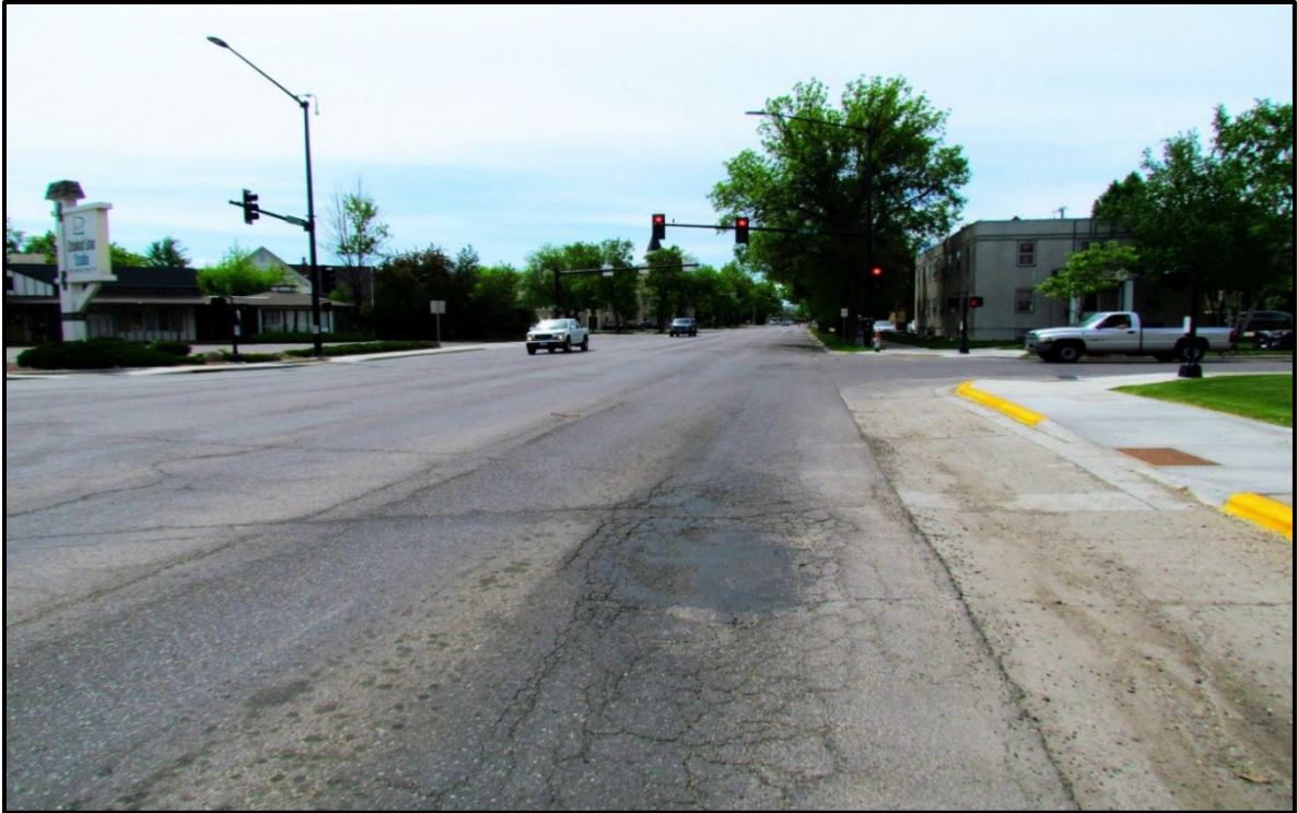
↑ Representative pavement distress in areas on Division St. of fatigue cracking (view south near Lewis Ave).
