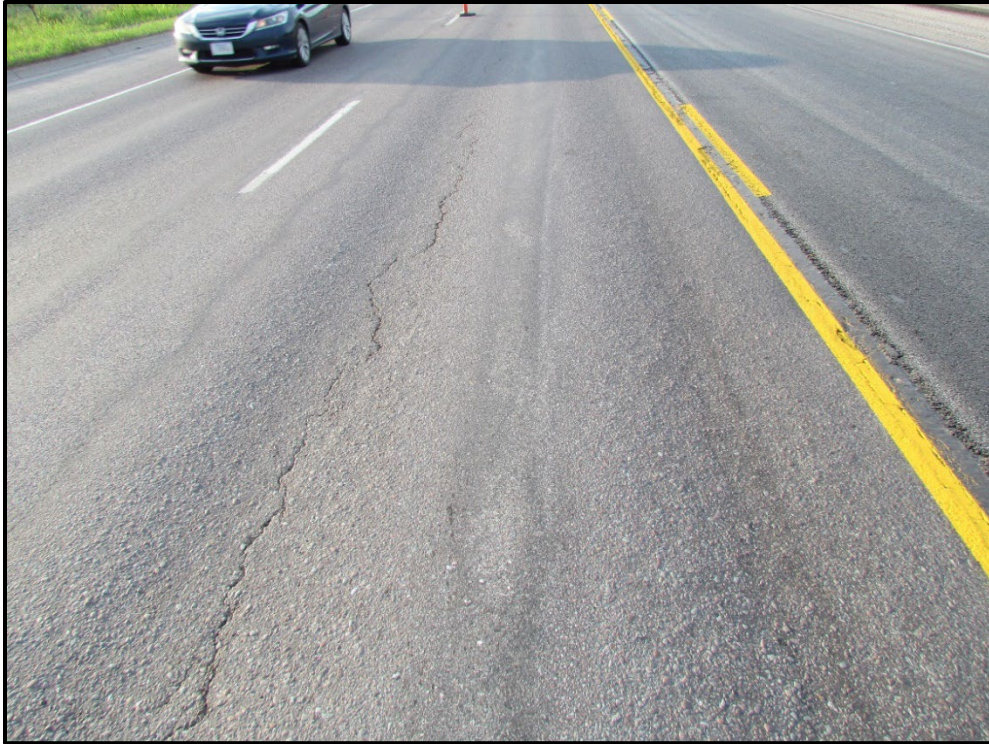
↑ Example of preconstruction conditions. There was a fair amount of longitudinal and transverse cracking.
