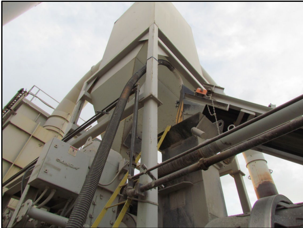
↑ The feeding tube was incorporated to the hot plant where the RAP belt deposited to the mixing drum.
