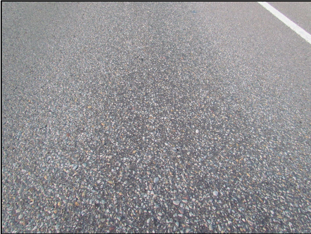
↑ Close up view of the southbound lane in the wheel path.
