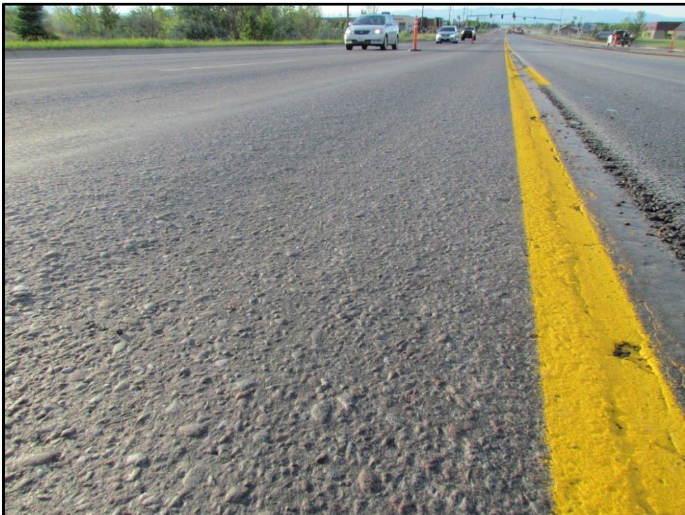
↑ Close-up view of the existing surface. There was significant wear and rutting.
