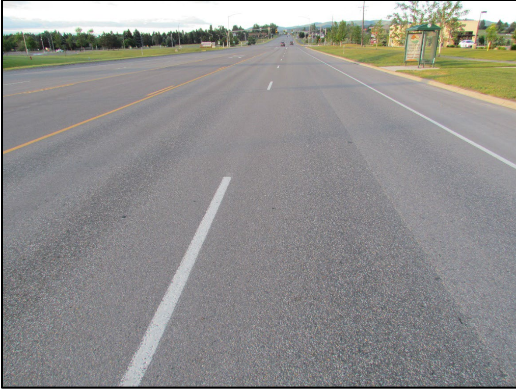
↑ View south of southbound lane. Nothing was noticed that wasn't ordinary pavement wear.
