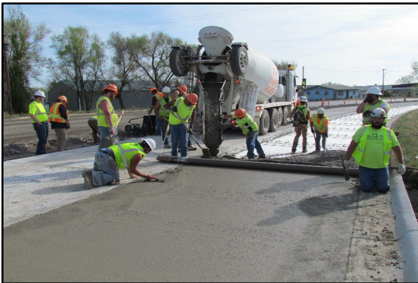
← Finishing the PCCP using a vibratory roller. This tool helps with maintaining a proper grade and cuts down on some hand work.
