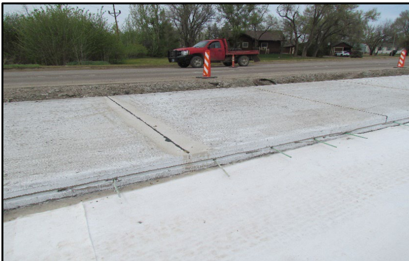
← Completed PCCP lane with rebar inserted and prepared bondbreaker in the other lane.
