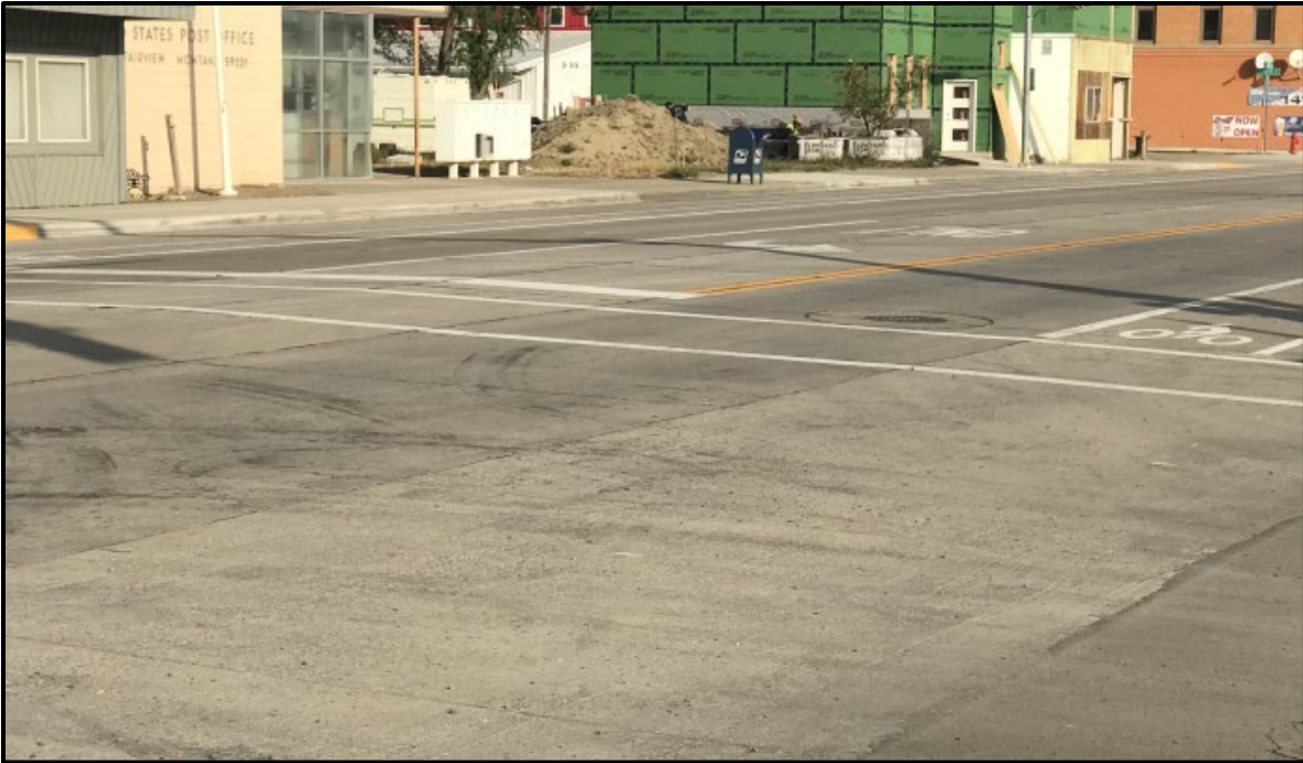
↑ Intersection of MT Hwy 200 and 6 th St N, view west. Test Section.
