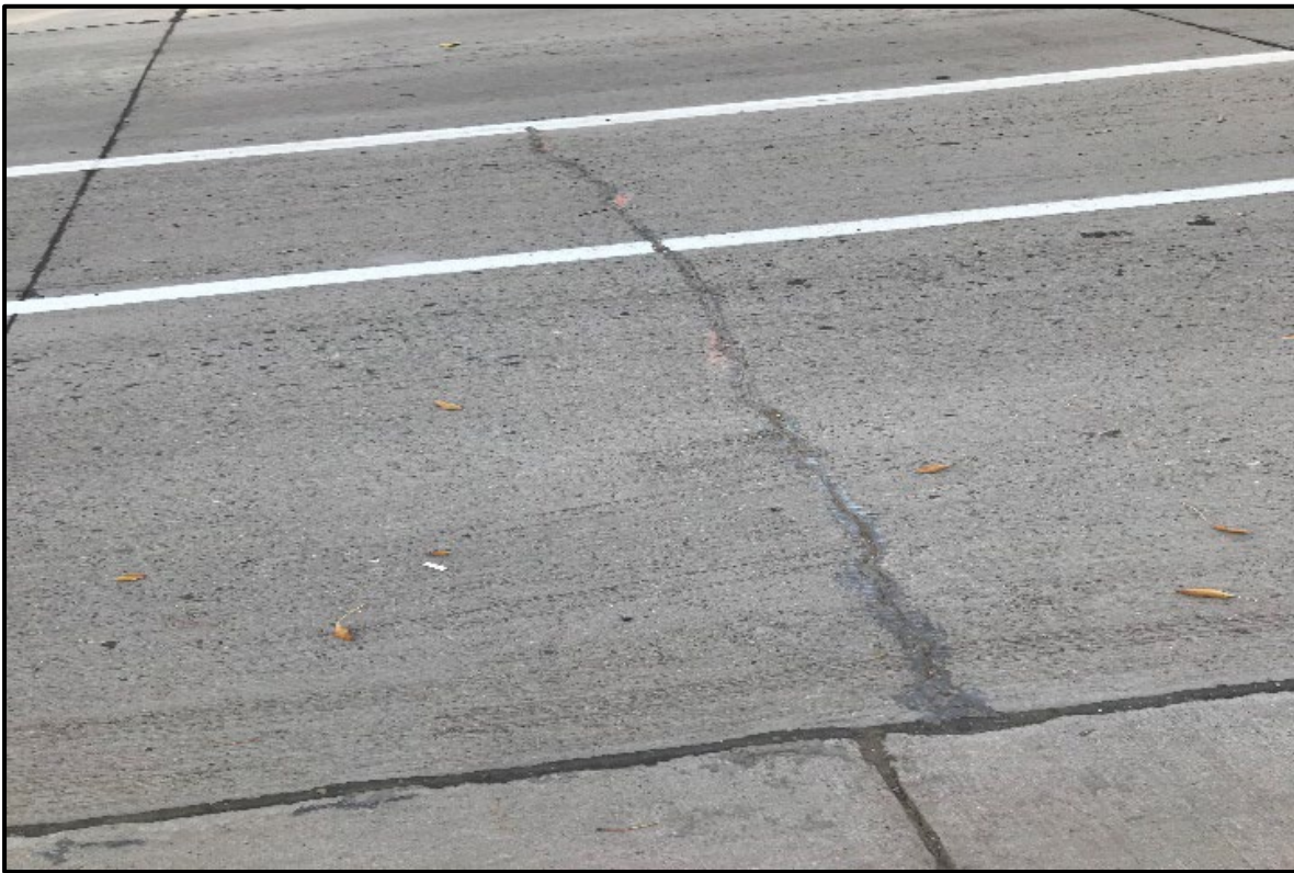
↑ Example of a crack that developed during curing process. Crack was sealed. No issues in compressive strength test results and no on-site material issues reported.
