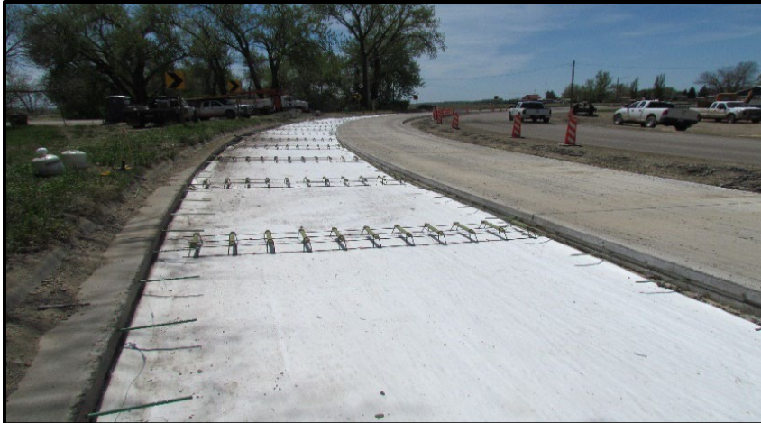
← Prepared SKAPS GT116 bondbreaker over CTB with a completed PCCP lane to the right. Also, example of dowl bar layout.
