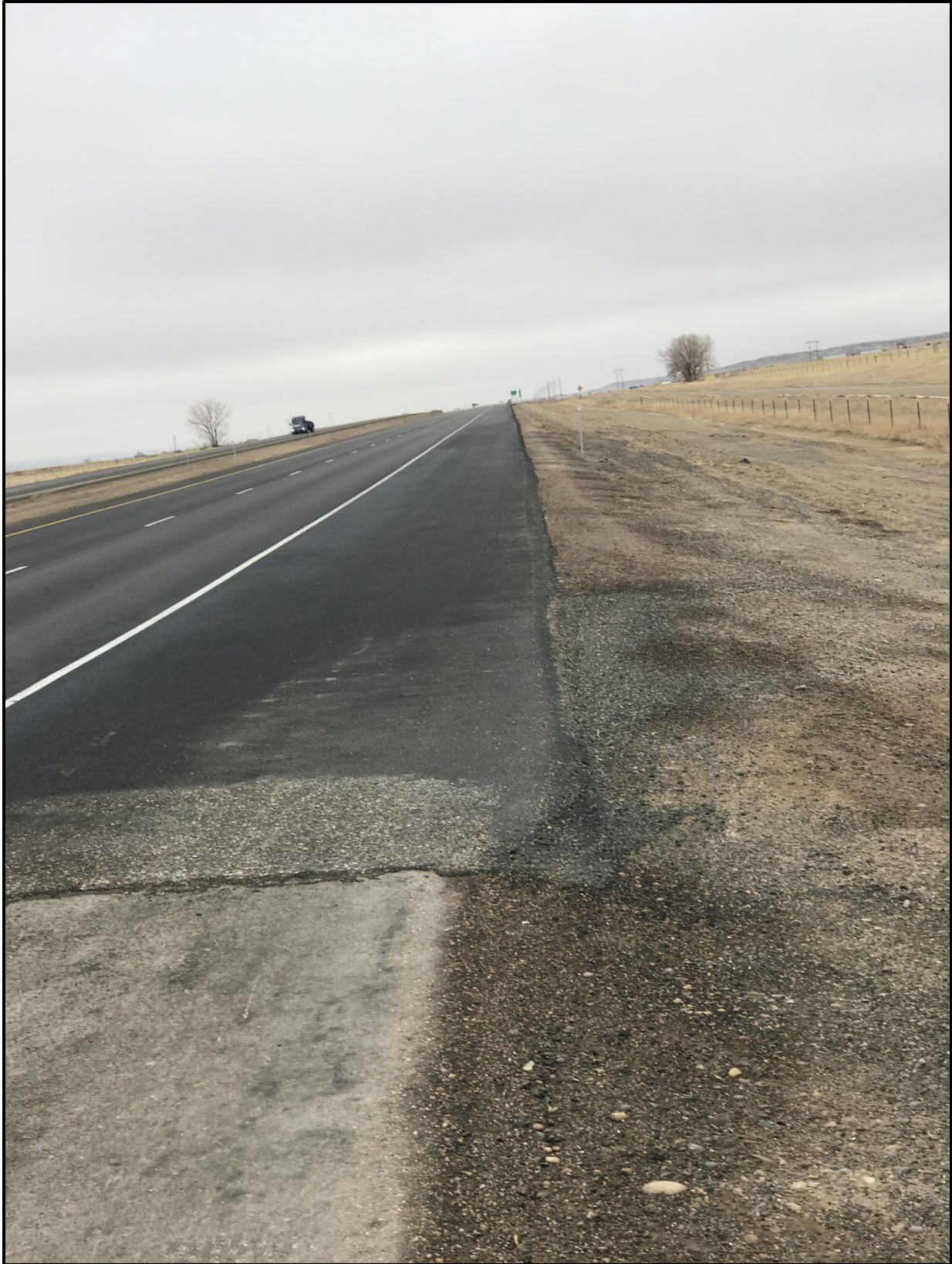
↑ RP 199.20, view west. Westbound shoulder, east end of the project, test section.
