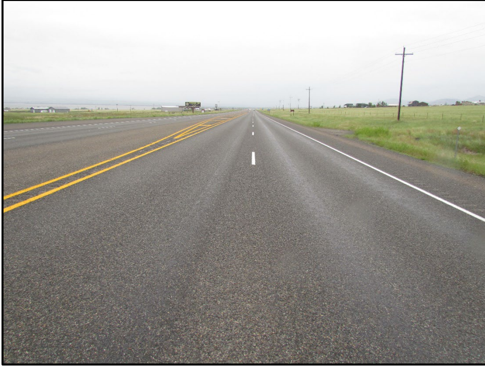
↑ RP 70.0, view south. This section is in the road smoothed section. Some wheel path wear can be seen.
