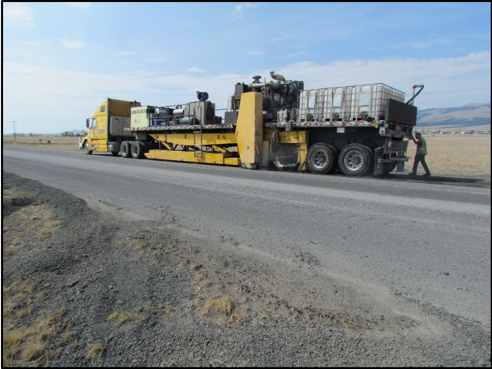
↑ Diamond grinding operation in action. The yellow level arms take in information and feed it to the on-board computer that controls the mill head.
