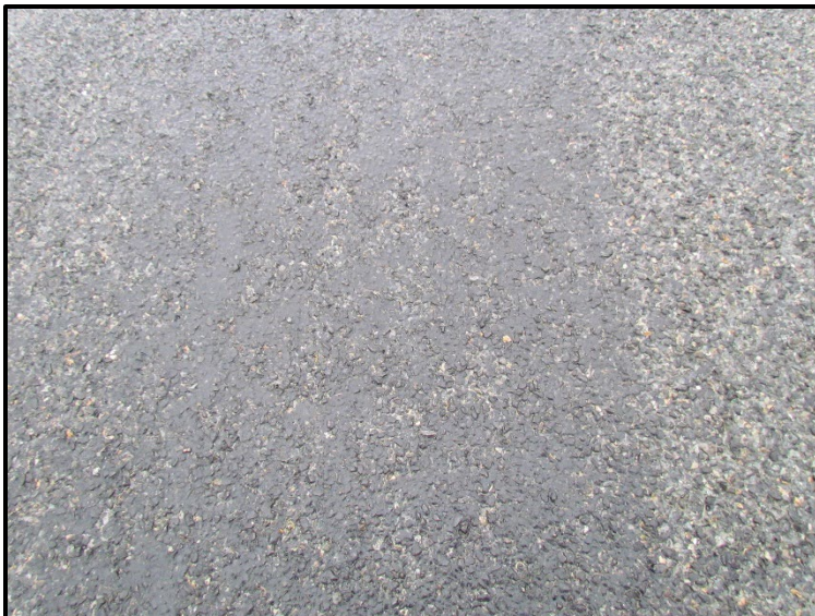
← Close-up of an area that the chip emulsion bled through the chips. This happened in multiple locations throughout the project.
