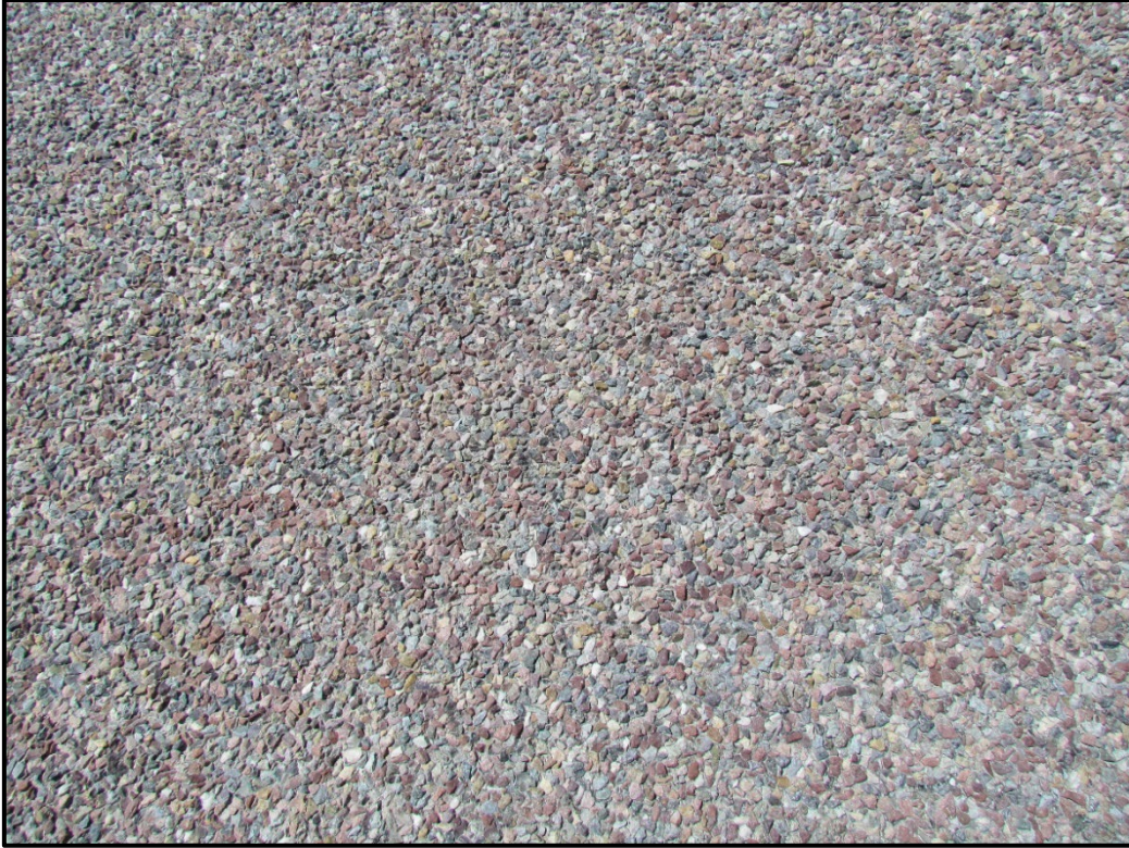
↑ RP 111.8, CHFRS-2P section, close-up of the chip seal surface.
