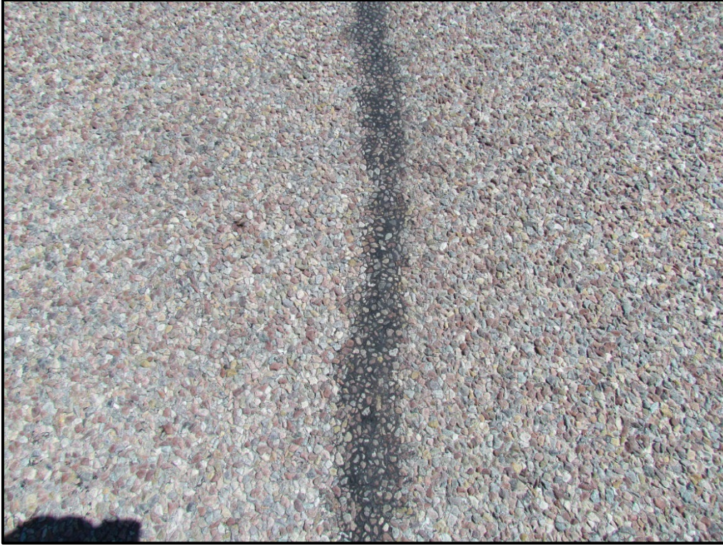
↑ RP 108.5, CHFRS-2P section, good example of crack seal bleeding. There doesn't appear to be any chip loss.
