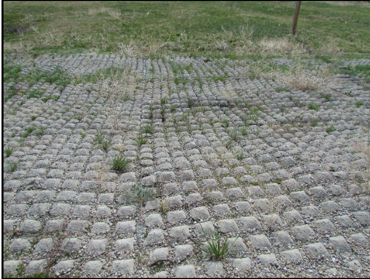
← View of some of the vegetation that has begun to grow through the Flexamat. Note that the bottom half of the ditch has more growth than the top.
