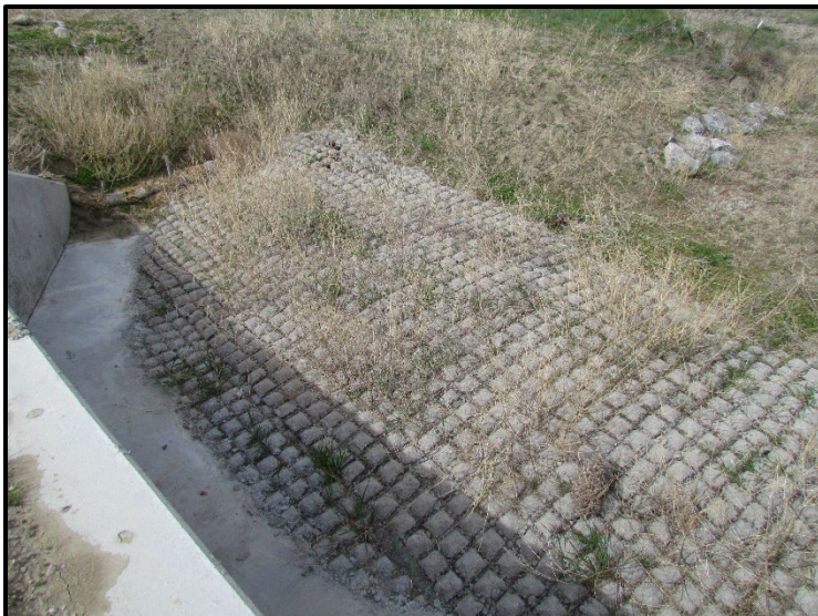
← Inlet side of the box culvert with noticeable plant growth through the Flexamat.
