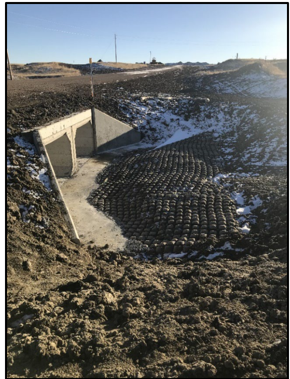
↑ Flexamat was also placed at the inlet and outlet of the box culverts.
