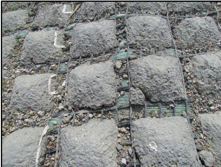
← Close-up view of the concrete blocks and geogrid making up the Flexamat in the outlet ditch. A few damaged blocks were noticed, most likely from installation.
