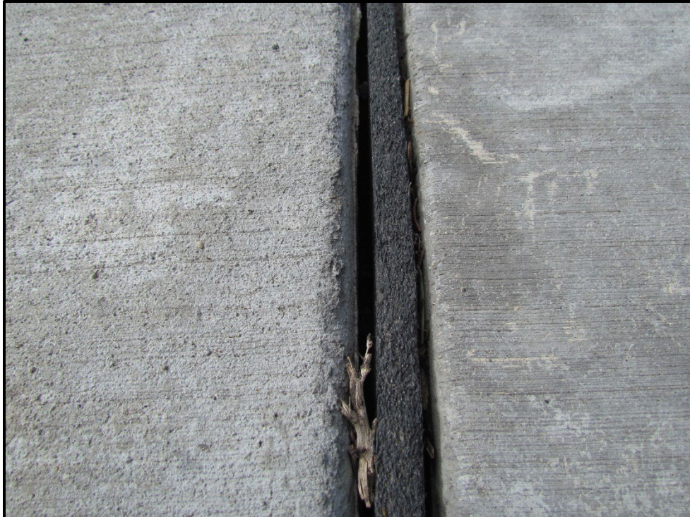
↑ Close-up view of the area of Nomaflex joint filler to be monitored due to the lack of contact with the concrete.
