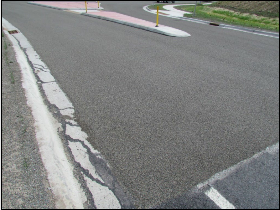
↑ Closer view of polymer overlay in northbound exit onto Spring Creek Road.
