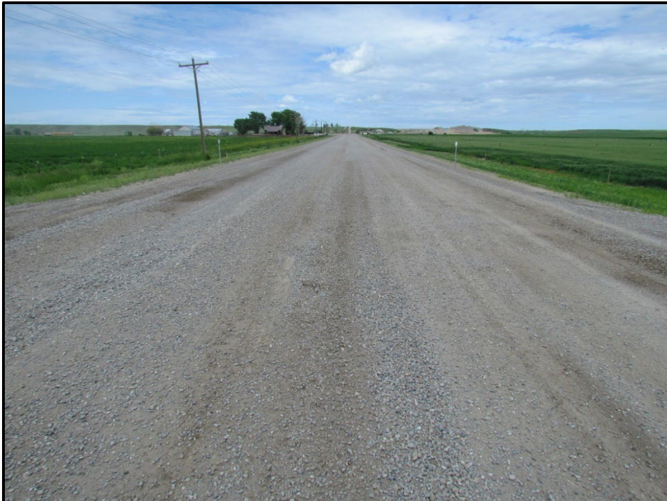
↑ Between stations 343+17 (south end of project) to 196+23, geogrid, fabric and CAC work was completed in the late summer and fall of 2021. This is an example of that section near station 275+00, view south. Per the MDT inspection crew, the material held up well through the winter and snowplow activities.
