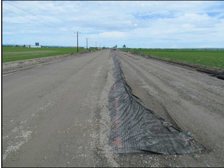
↑ Completed southbound lane of CAC surfacing after spreading and during compaction. Note that enough grid was exposed to meet the 24" overlap required in the special provisions. Near station 90+00, view north.
