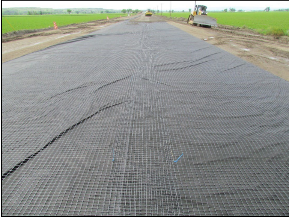
↑ View of the geogrid and fabric. Note that the grid was being tied together with zip ties and laid in accordance with the special provision. Every 10' on the longitudinal joint and 4' for transverse joints. Near station 82+00.
