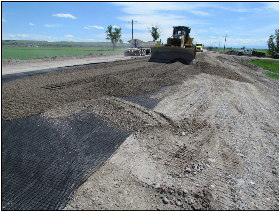
↑ The contractor opted to use a dozer for CAC placement rather than a grader to avoid causing damage due to excessive tire activity on the geogrid. Near station 78+00.
