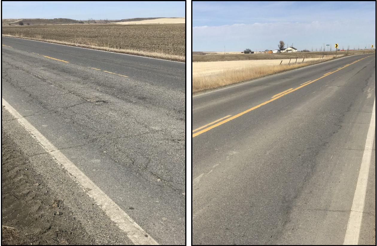
↑ Examples of preconstruction roadway conditions. Left photo is view south and right is view north. There is heavy rutting as well as longitudinal and transverse cracking. Per the project manager, the northbound lane experiences higher amounts heavy commercial truck traffic due to sugar beet operations in the area.
