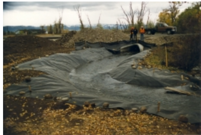
Synthetic liners can be used to minimize soil erosion during construction (BMP SS-7).
