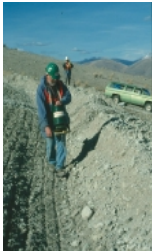
Temporary seeding is used to stabilize soils through new plant growth (BMP SS-4).
