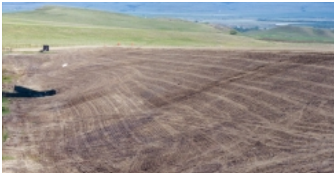
Soil Roughening reduces runoff velocity, increases infiltration, reduces erosion, traps sediment, and prepares soil for seeding and planting by giving seed an opportunity to take hold and grow (BMP SS-12).
