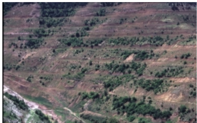
Terraced slopes help reduce velocities and allow deposition of sediment on the terraces. Steep slope revegetation can be a difficult task (BMP SS-13).
