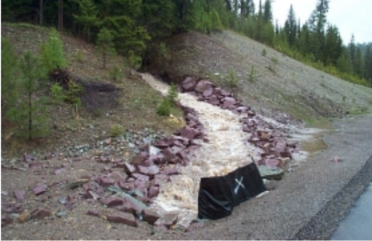
Rock Lined channels are a method of conveying discharges with a minimum of soil erosion (BMP SS-9).
