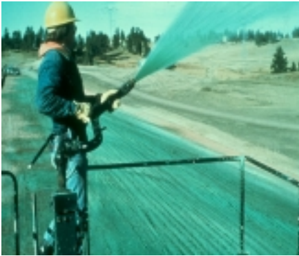
Soil binders and hydraulic mulch are used to stabilize soils (BMP SS-3).
