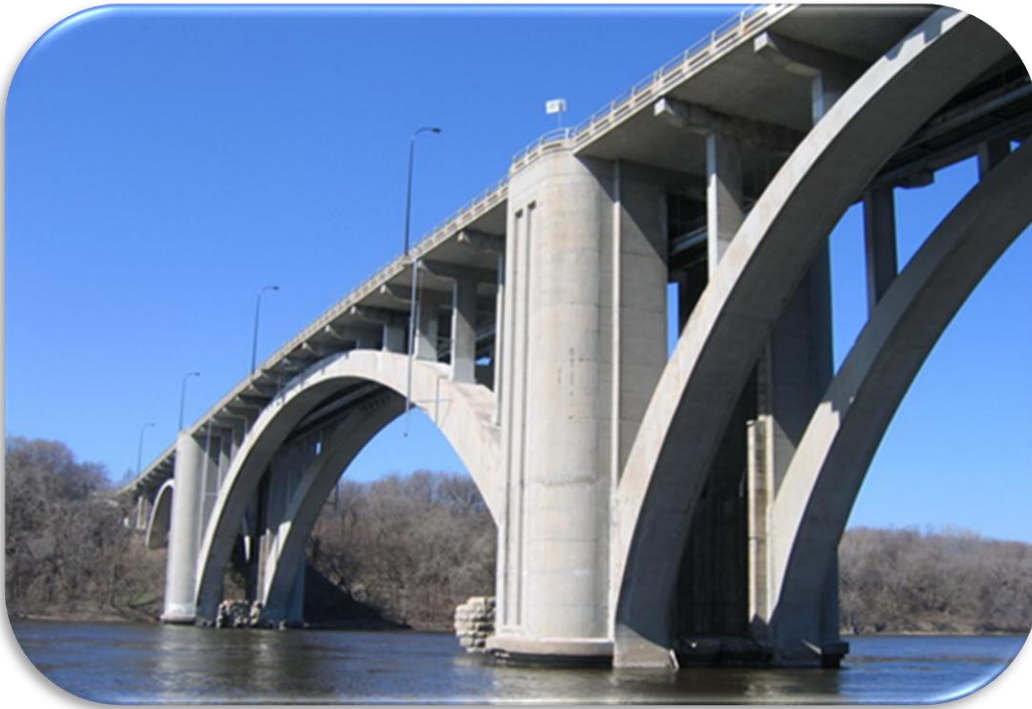
Figure 1. WJE developed the repair and rehabilitation procedures for the historic preservation of the Franklin Avenue Bridge in Minneapolis, MN.
