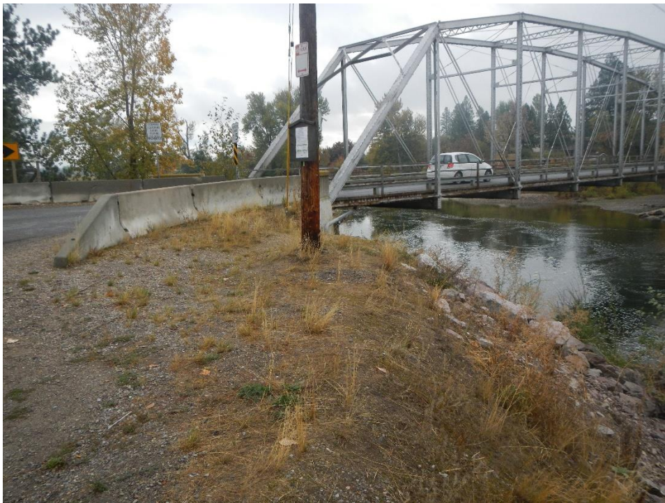
Photo 2: Maclay Bridge and the west approach and abutment area, view from the shoulder of River Pines Road
