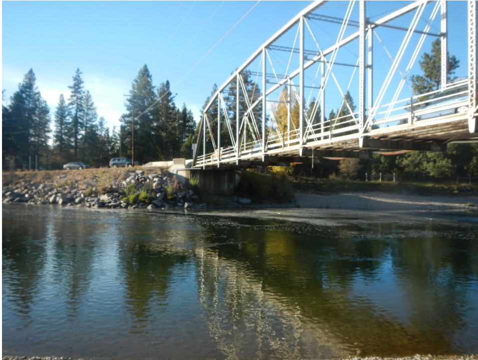
Photo 1: Maclay Bridge and the west approach and abutment area, view from the Bitterroot River
