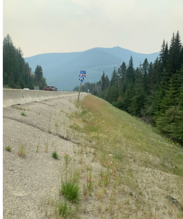
Photo 2: Near RP 0.3, looking east. Typical roadside environment with heavy sanding material, steep grades, visible erosion, and sparse vegetation.
