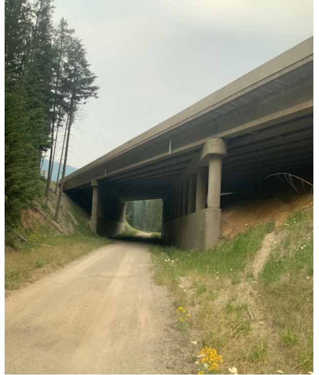
Photo 10: I-90 bridge with NORPAC road underneath, at RP 5.1. Note wildlife trail under bridge to right of roadway.
