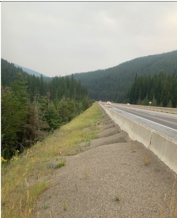
Photo 3: Near RP 1.7, looking east. Typical roadside environment with heavy sanding material, steep grades, visible erosion, and sparse vegetation.
