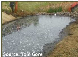
Properly-installed sediment traps will include an armored weir with a low point for discharge.
