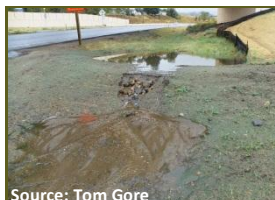
Lack of an armored weir will lead to failure/erosion at the discharge location.
