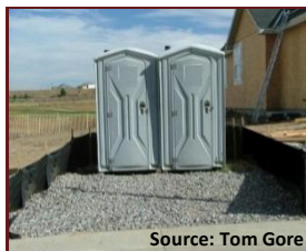
Station portable toilets in designated staging areas.
