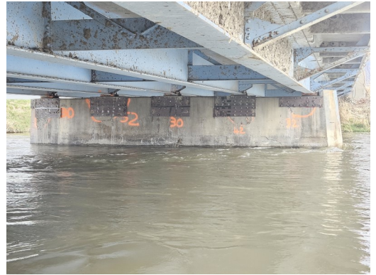
Pictured above: The completed bridge repairs on Saturday after cleanup of the site was complete.
