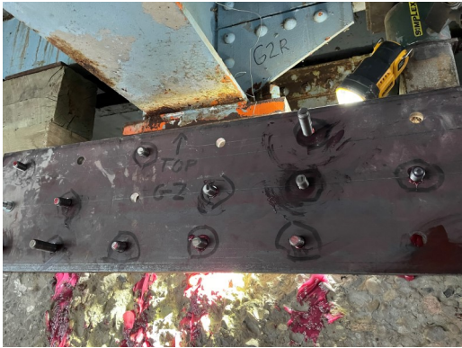
Pictured above: Example of repair progress at the end of the first night (Thursday) - some steel plates have been anchored and epoxied on the pier.
