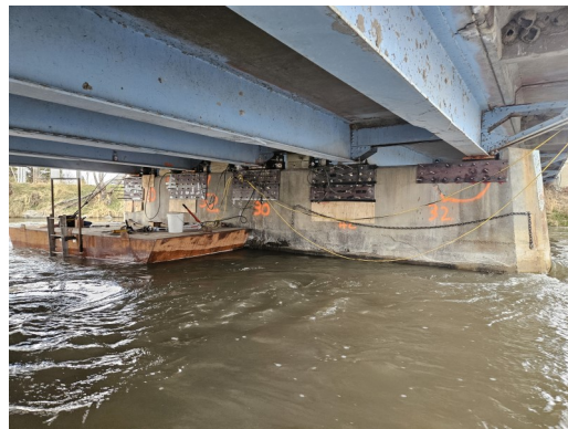
Pictured above: Bridge repairs near completion on Friday, with some beam sets finished and some waiting for epoxy to dry before finishing.
