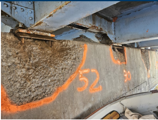
Pictured above: The pre-repair condition of the bridge's concrete cap shows the loss of support under the girder bearings.
