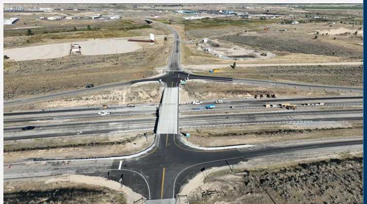
Aerial view of the Silver Bow interchange bridge deck replacement near the junction of I 15 and I 90 near Butte
